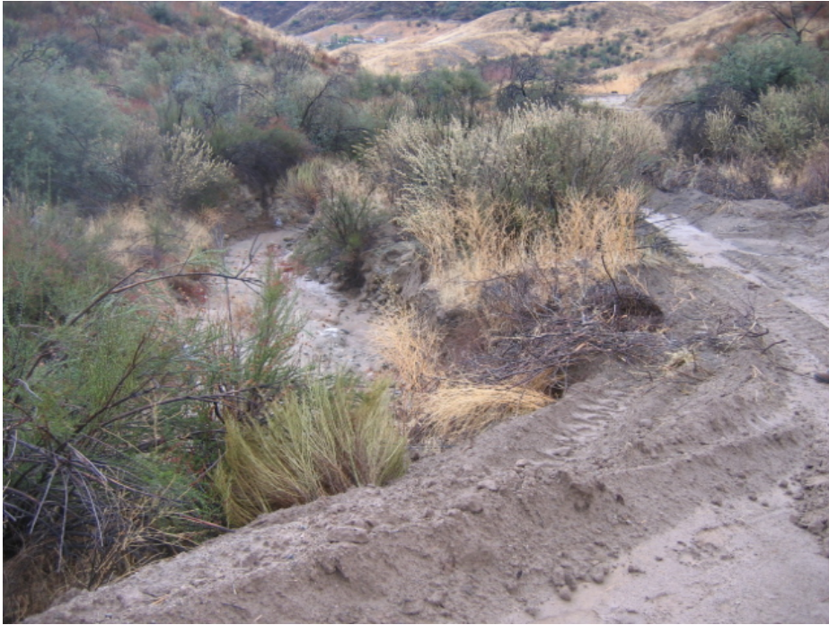
Figure 1: Recent ground disturbing activities near NC 28 on Section 1 have not been fortified with BMPs to prevent loose soils from eroding outside of the project area. The CPUC EM has reminded Burns & McDonnell Environmental staff that BMP installation is required in areas of ground disturbance.
