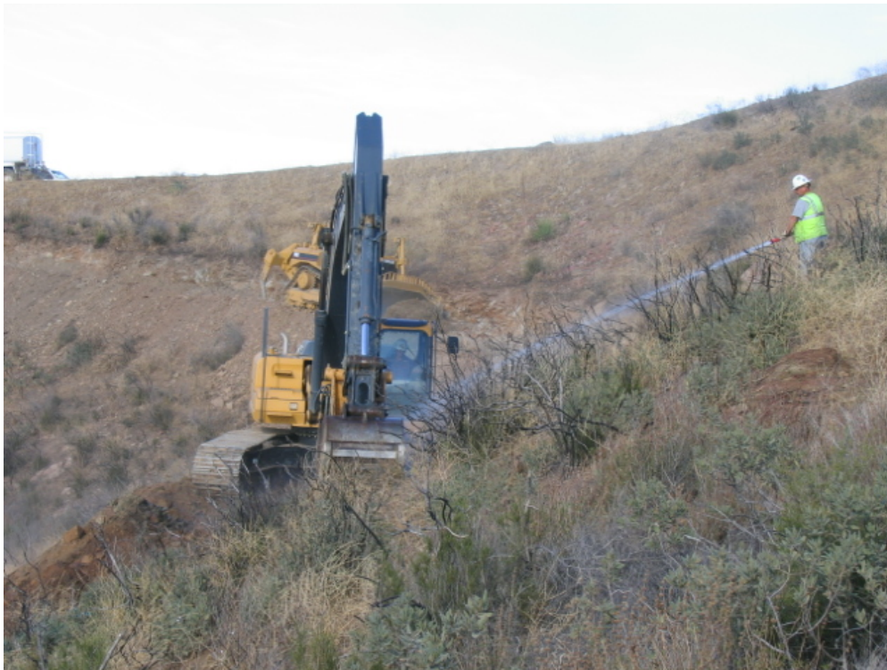
Figure 4: Temporary road construction to access Tower 41. An excavator was used to cut the new road. Topsoil was separated in areas of less than 40% slope.
