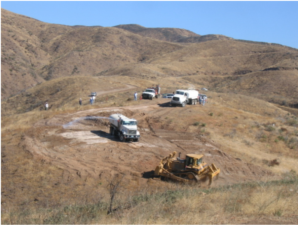
Figure 3: Grading of a wire stringing site near Tower 33 in the ANF took place without topsoil segregation. The ANF Construction Plan required soil segregation in areas of less than 40% slope for restoration purposes.
