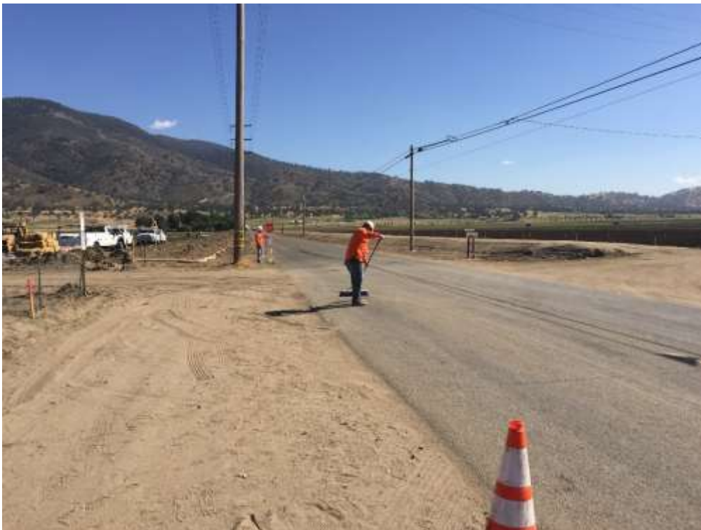
Figure 2 – Manual street sweeping was conducted along Pelliser Road while the stabilized construction entrance was being constructed, July 26, 2017.
