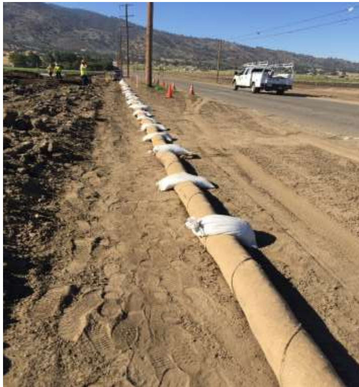
Figure 3 – Erosion control BMPs were observed to be incorrectly installed along Pelliser Road July 26, 2017.
