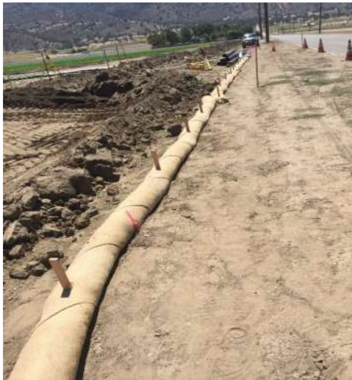
Figure 4 – Construction crews were alerted to the incorrect BMP installation and repairs were immediately made, July 27, 2017.
