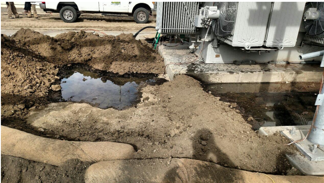
Figure 2 – Approximately 125-gallons of mineral oil spilled onto the ground under the damaged transformer. Photo courtesy of SCE.
