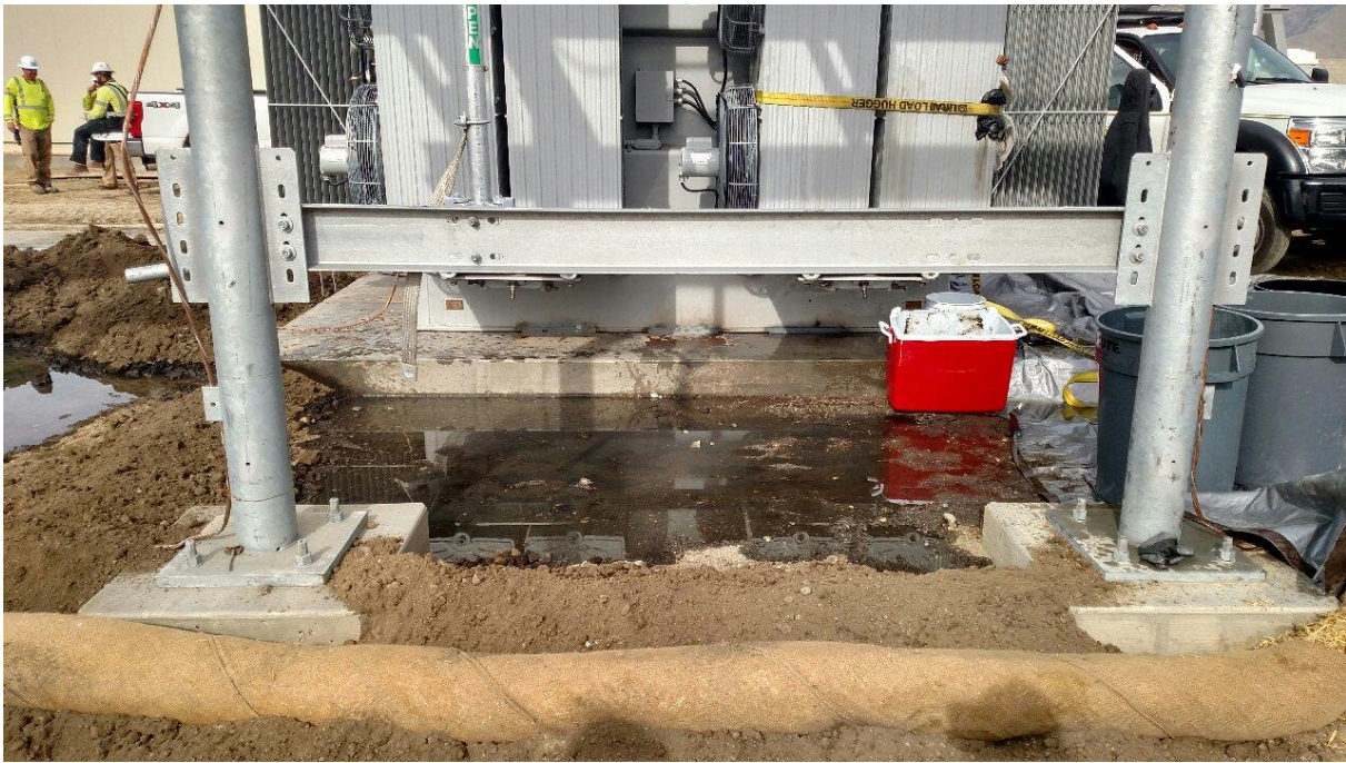
Figure 3 – Containment around the damaged transformer to prevent the spill from spreading. Photo courtesy of SCE.
