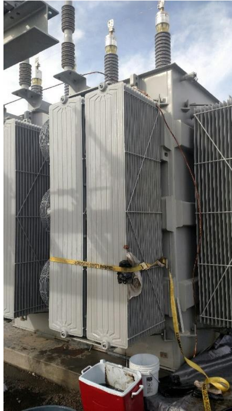
Figure 1 – Henkels and McCoy crew inadvertently damaged Transformer #1 causing a mineral oil spill at the substation site. Photo courtesy of SCE.
