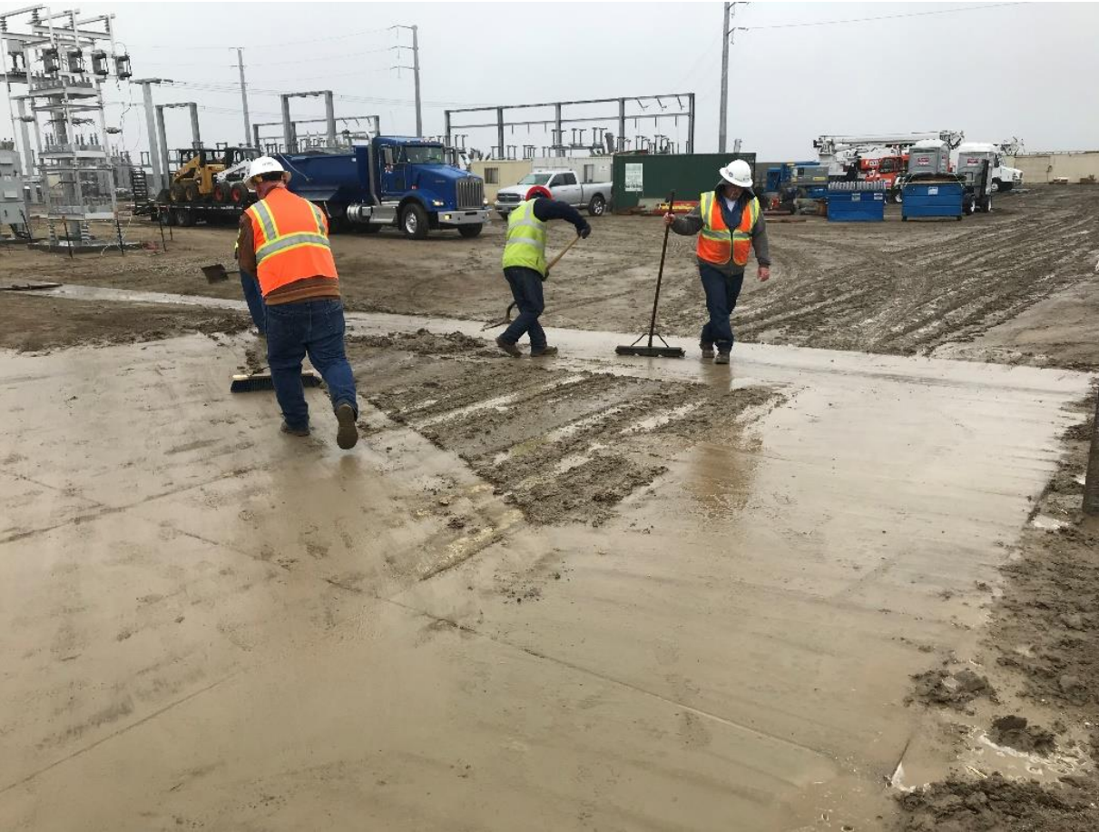
Figure 4 – Crews using brooms to clean off mud from the substation entrance. Work was called off later due to rain.
