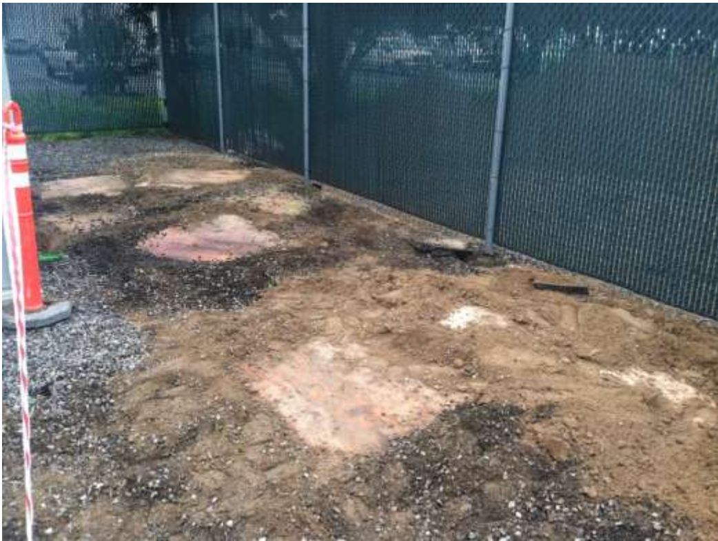
Figure 7 – Augered holes are secured and sealed at the Gallo Substation. View southeast, 01/20/15.
