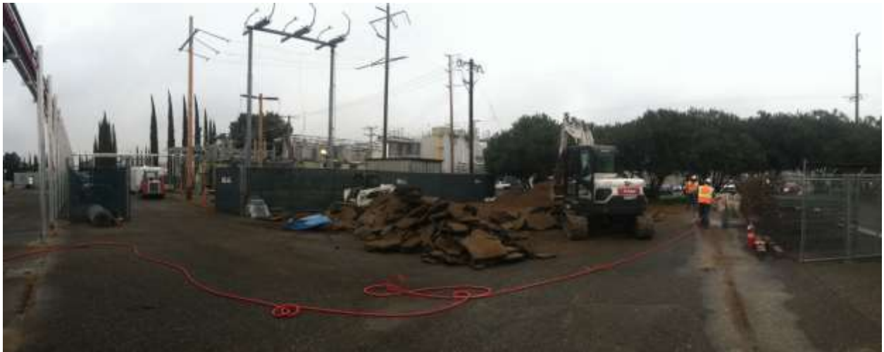
Figure 4 – Construction continued at the Gallo Substation during the subject period. View northeast from southwest corner of future substation area, 01/15/15 top, 01/20/15 bottom.
