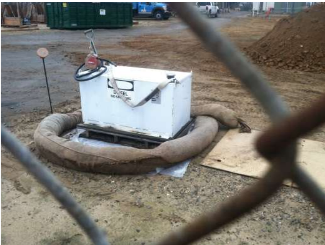
Figure 8 – Inadequate secondary containment was observed around a diesel storage tank. View northwest, 01/20/15.
