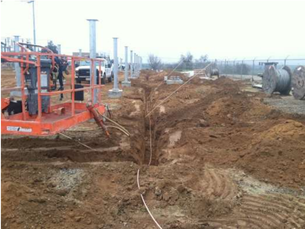
Figure 2 – Trenching and structure installation occurred at the Cressey Substation during the subject period. View southeast, 01/20/15.
