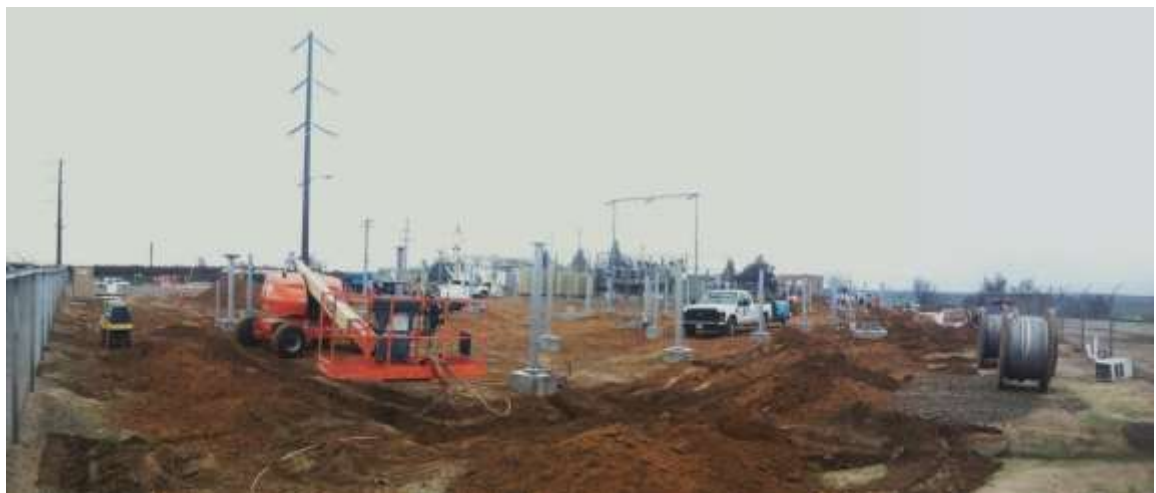
Figure 1 – Trenching and structure installation occurred at the Cressey Substation during the subject period. View from southeast corner of substation facing northwest, 01/08/15 top, 01/15/15 middle, 01/20/15 bottom.
