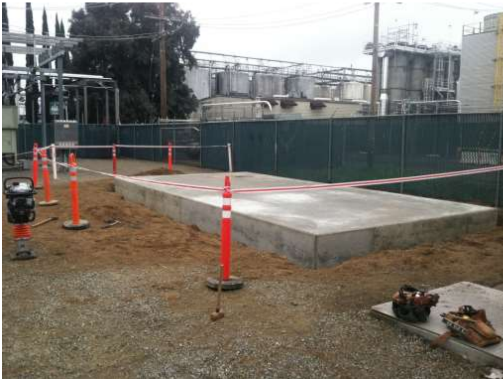
Figure 3 – Foundation installation occurred at the Gallo Substation during the subject period. View northeast, 01/20/15.
