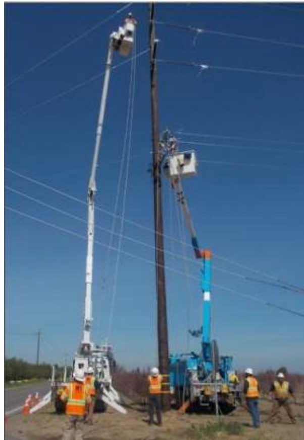
Figure 2 – Crews conducted pull and tensioning activities during the subject period. (Photo provided by PG&E).
