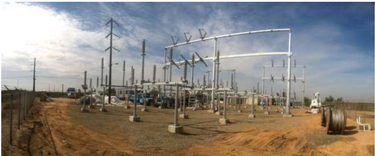
Figure 1 – Structure installation continued at the Cressey Substation during the subject period. View from southeast corner of substation facing northwest, 01/08/15 above 02/03/15 middle, 3/10/15 below.
