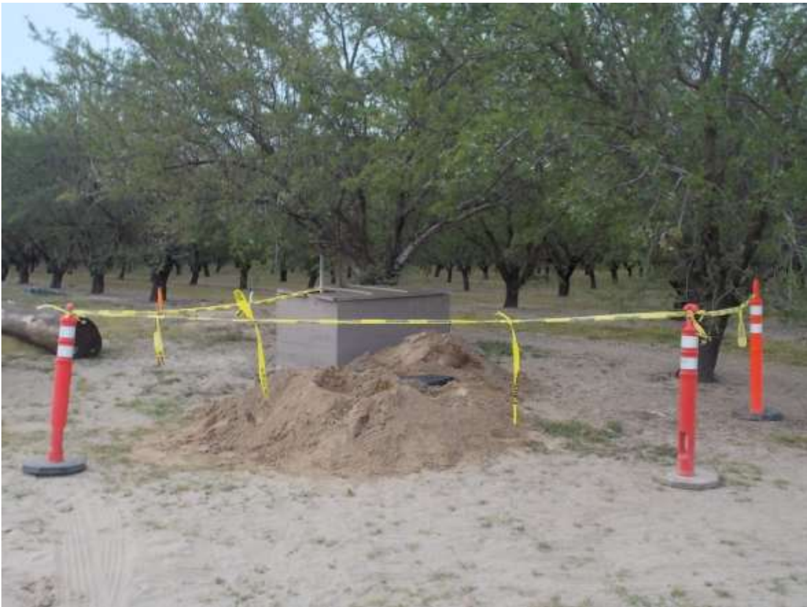
Figure 4 – To protect the public, project personnel installed safety flagging and cones around augered holes (following this photo, large gravel bags were also positioned over the holes). View near the corner of Robin Ave and Magnolia Ave, facing north east (Photo provided by PG&E).
