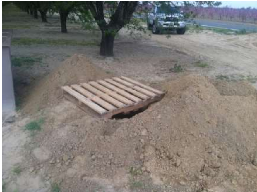
Figure 3 – Augered pole foundations were poorly covered by crews at the end of the day; however, compliance personnel corrected deficiencies. View near the corner of Robin Ave and Magnolia Ave, facing north.
