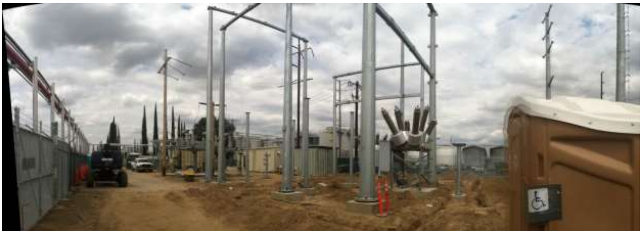
Figure 1 – Construction continued at the Gallo Substation during the subject period. View northeast from southwest corner of future substation area, 01/20/15 above, 02/03/15 middle, 05/21/15 below.
