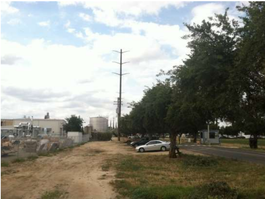
Figure 3 – Poles were installed at the Gallo Winery entrance during the subject period. View north, 5/21/15.
