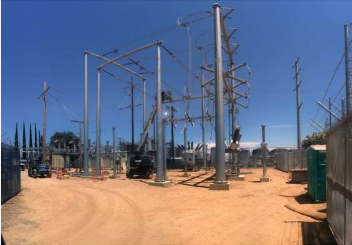
Figure 1 – Structure installation continued at the Gallo Substation during the subject period. View northeast, 6/12/15.
