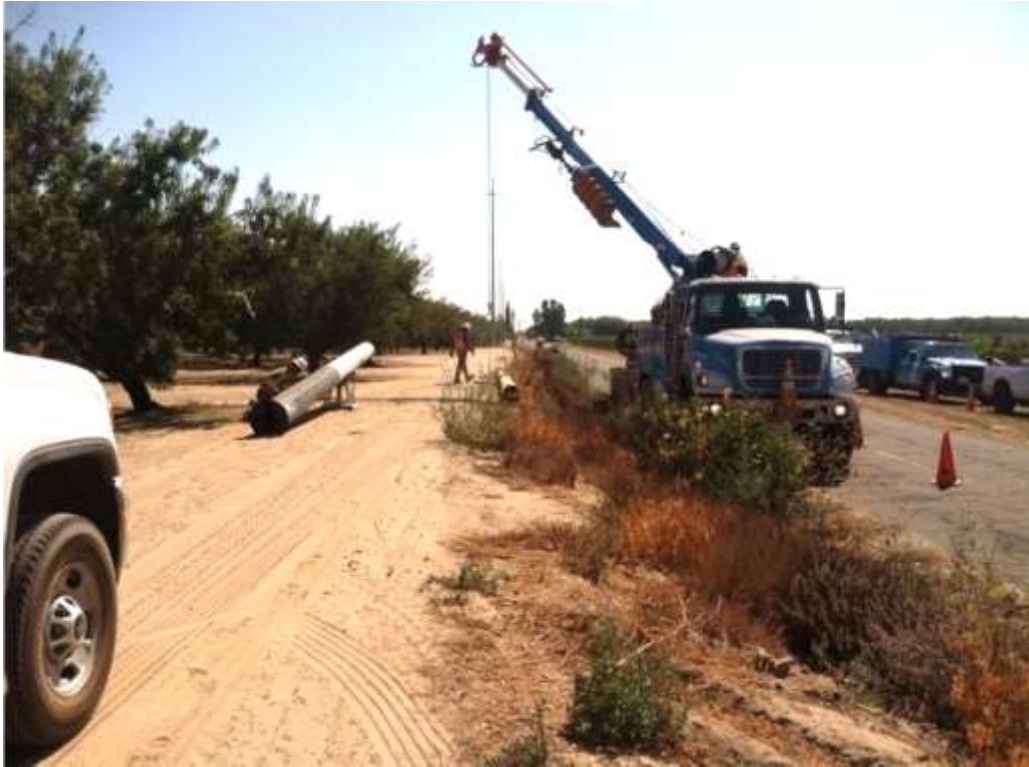
Figure 1 – Poles were installed along Magnolia Avenue during the subject period. View east. Photo provided by PG&E.
