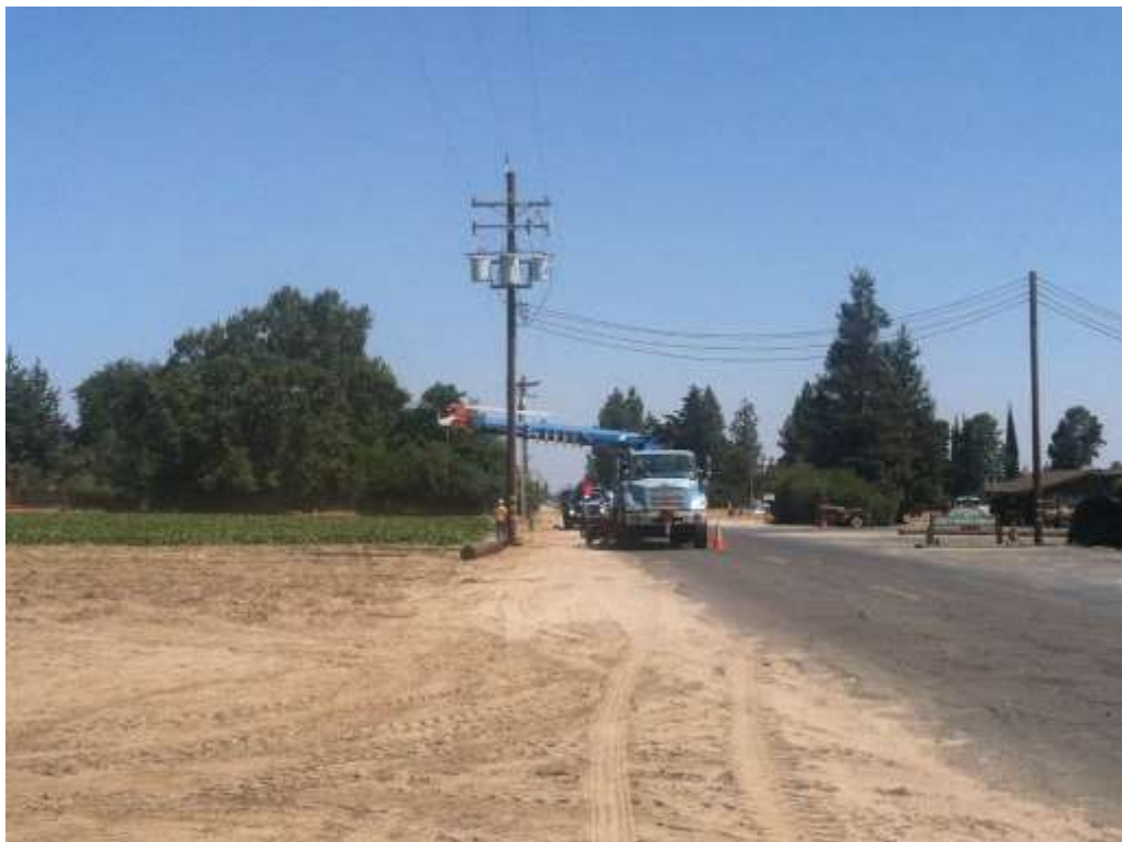
Figure 2 – Crews staged poles along Magnolia Avenue during the subject week. View west 9/1/15.
