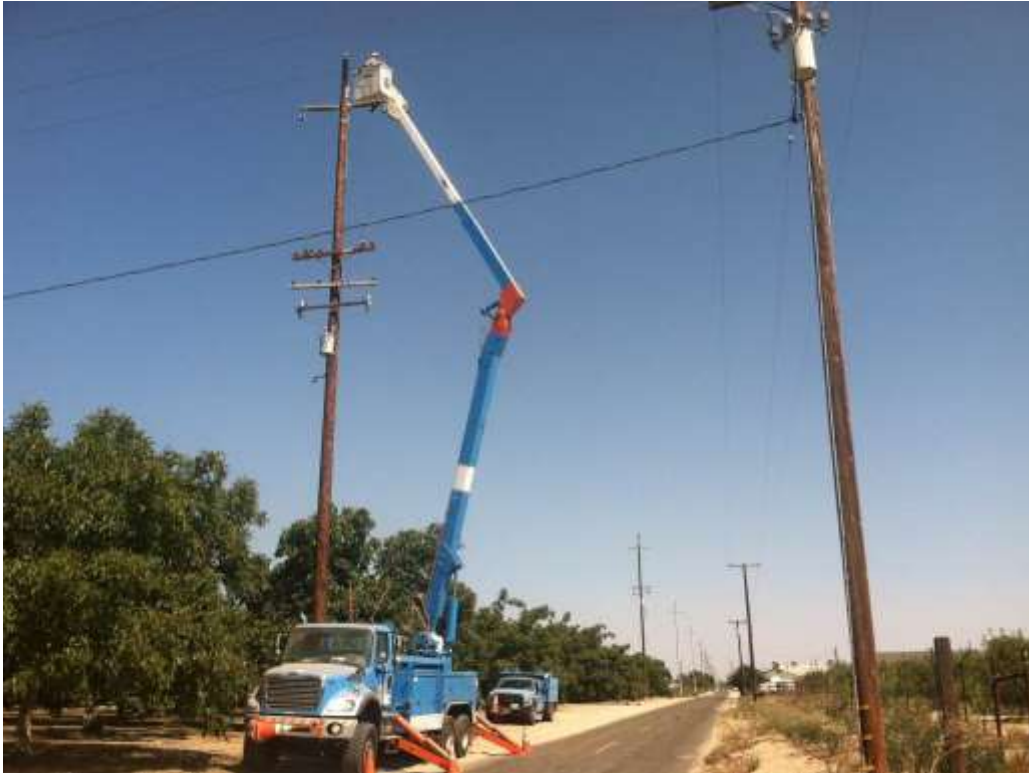
Figure 1 – Crews installed components on transmission poles during the subject period. View east 9/1/15.
