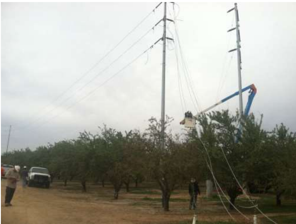
Figure 2 – Crews installed wire along the reroute portion of the alignment during the subject period. View northwest, 10/27/15.
