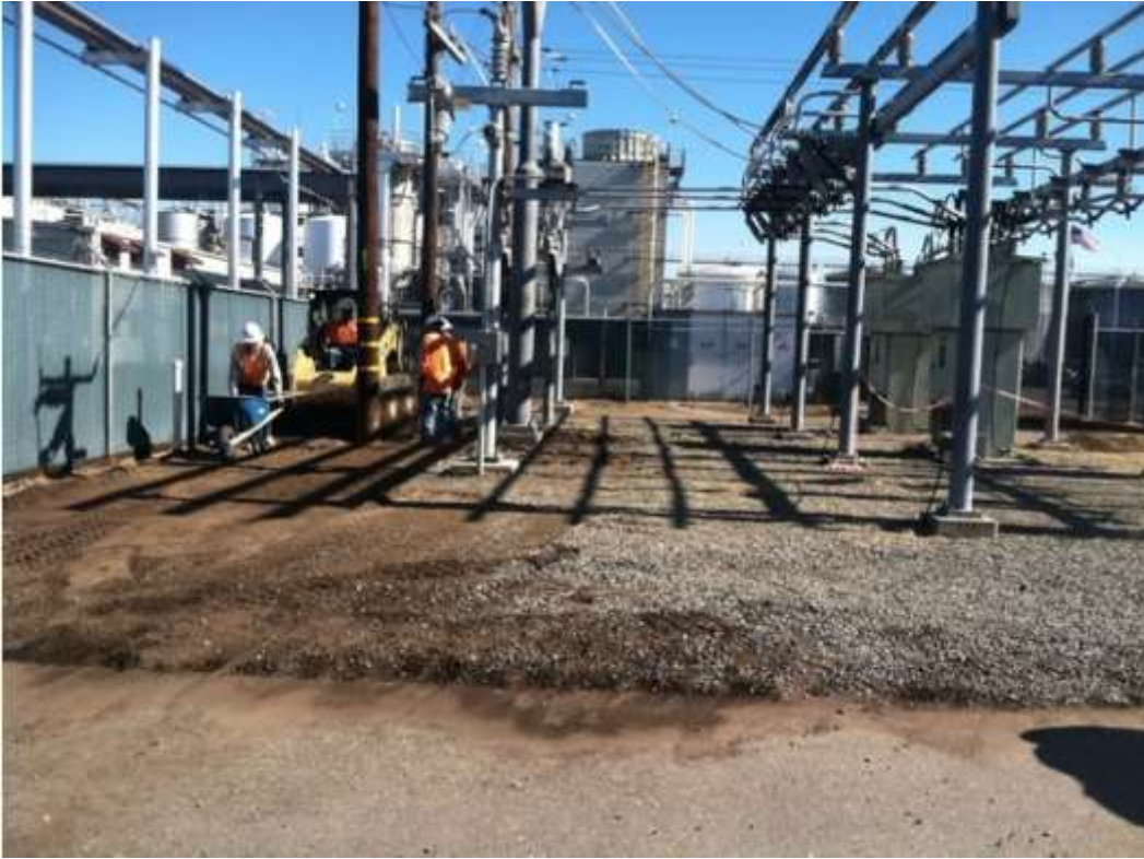
Figure 1 – Minimal construction activities occurred at the Gallo Substation during the subject period. View east (Photo provided by PG&E).
