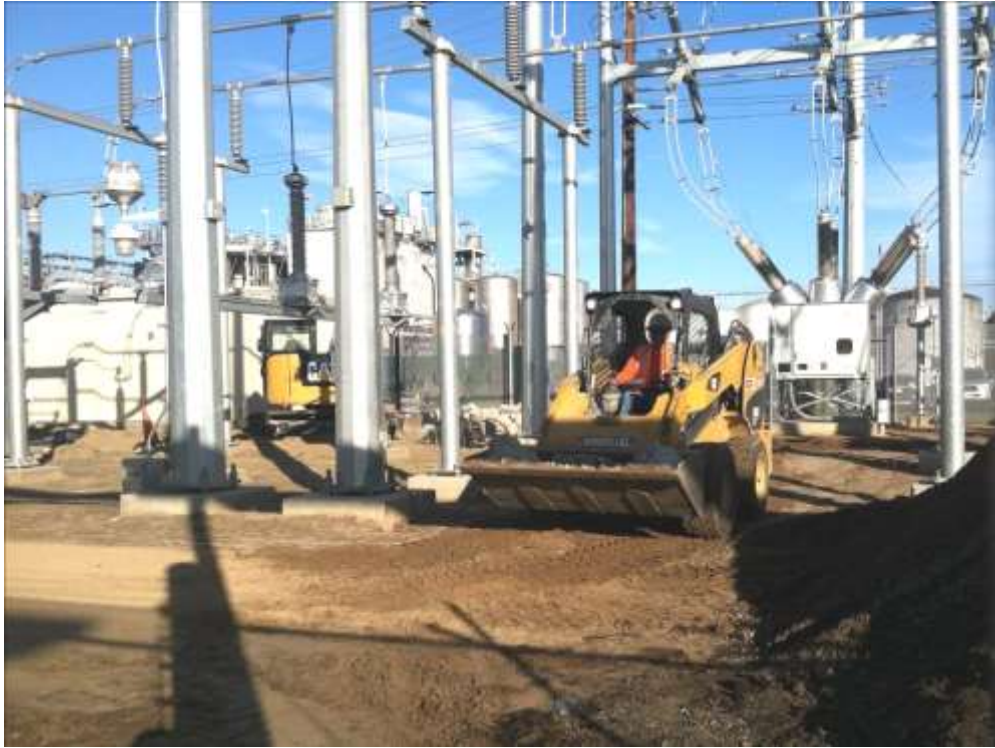
Figure 1 – Demolition activities occurred at the Gallo Substation during the subject period. View northeast, 11/4/15.
