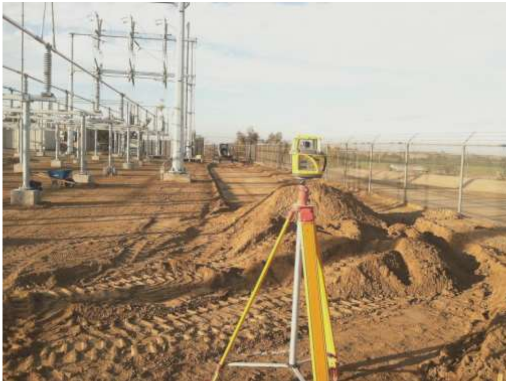
Figure 2 – Crews conducted grading activities at the Cressey Substation during the subject period. View north, 11/4/15.
