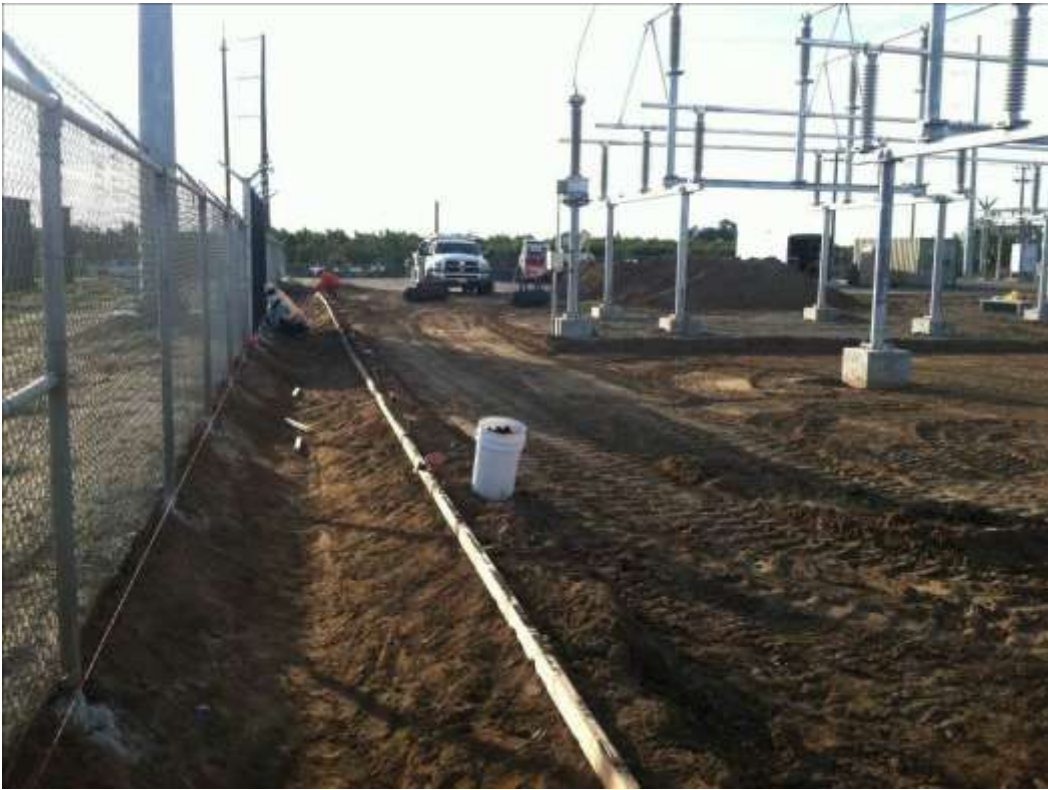
Figure 3 – Crews framed the drainage culvert for the Cressey Substation during the subject period. View west, 11/4/15.
