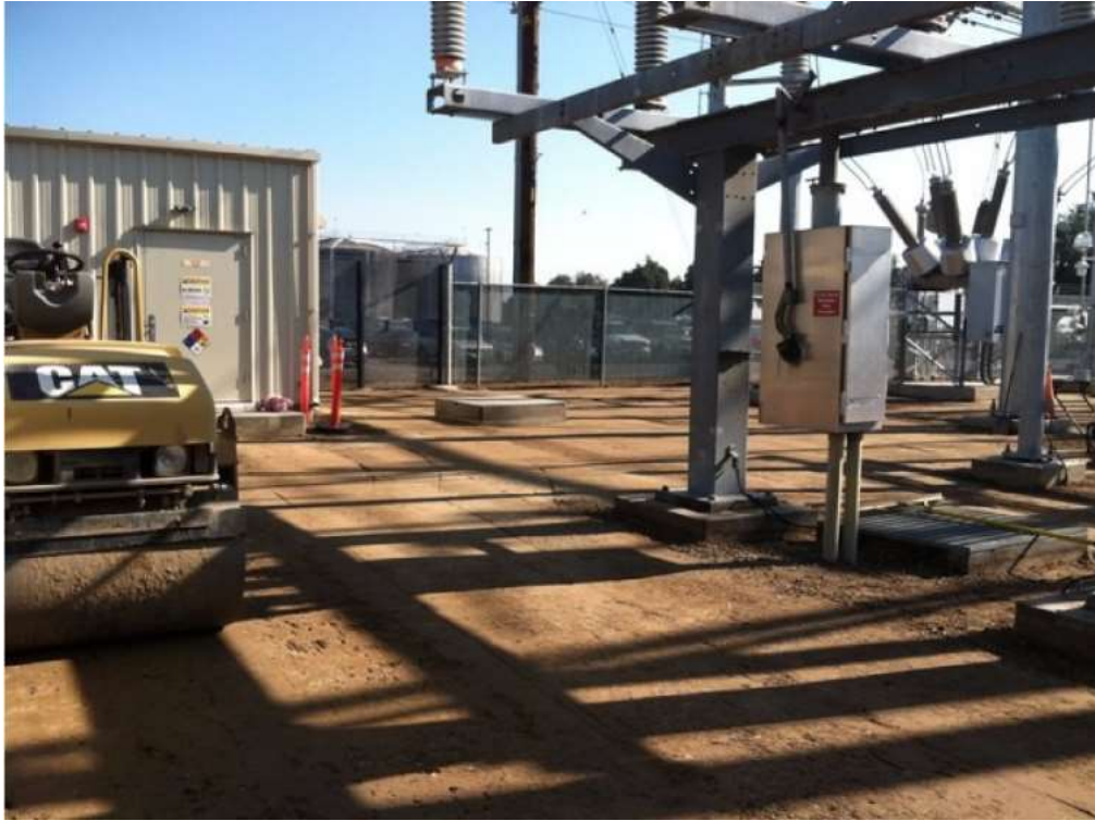
Figure 1 – Grading and paving activities occurred at the Gallo Substation during the subject period. View southeast (Photo provided by PG&E).
