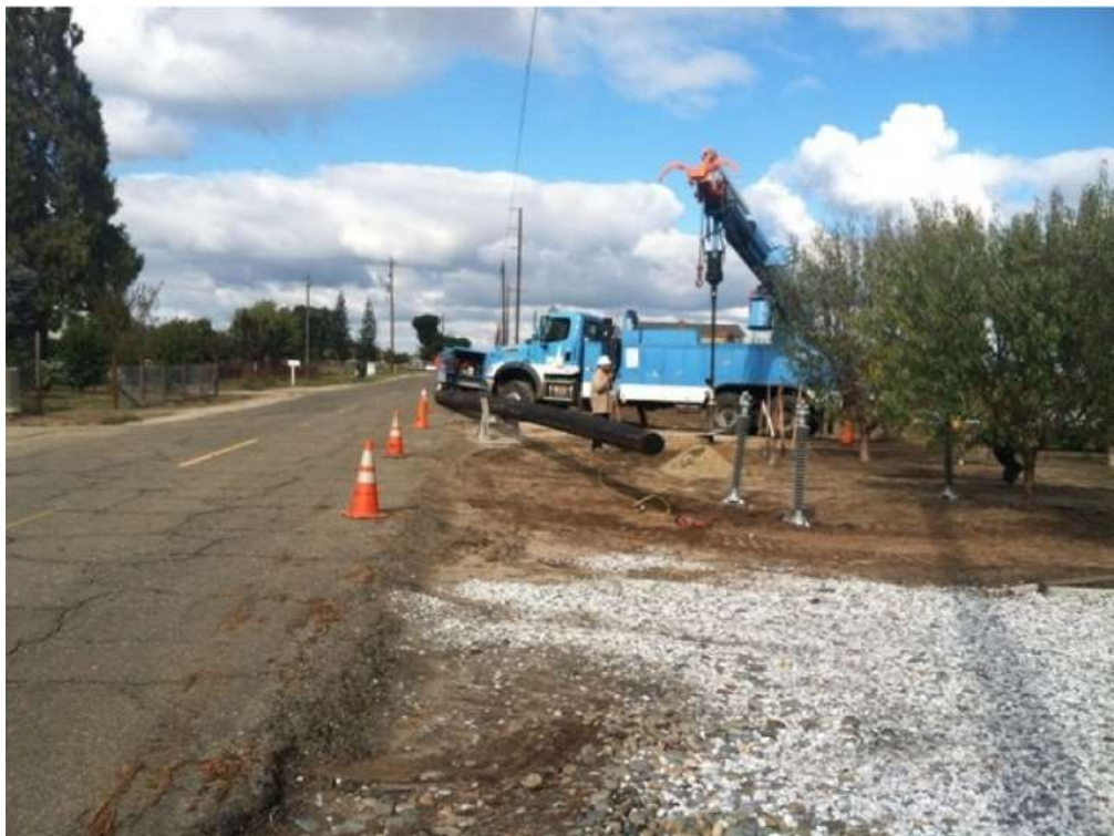
Figure 2 – Crews installed poles along sections of the alignment during the subject period. View north (Photo provided by PG&E).
