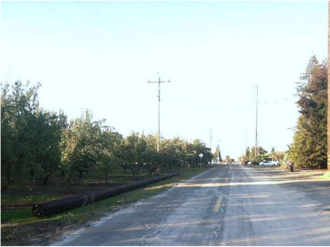
Figure 3 – Poles remain staged along the alignment in anticipation of continued work. View north, 11/11/15.
