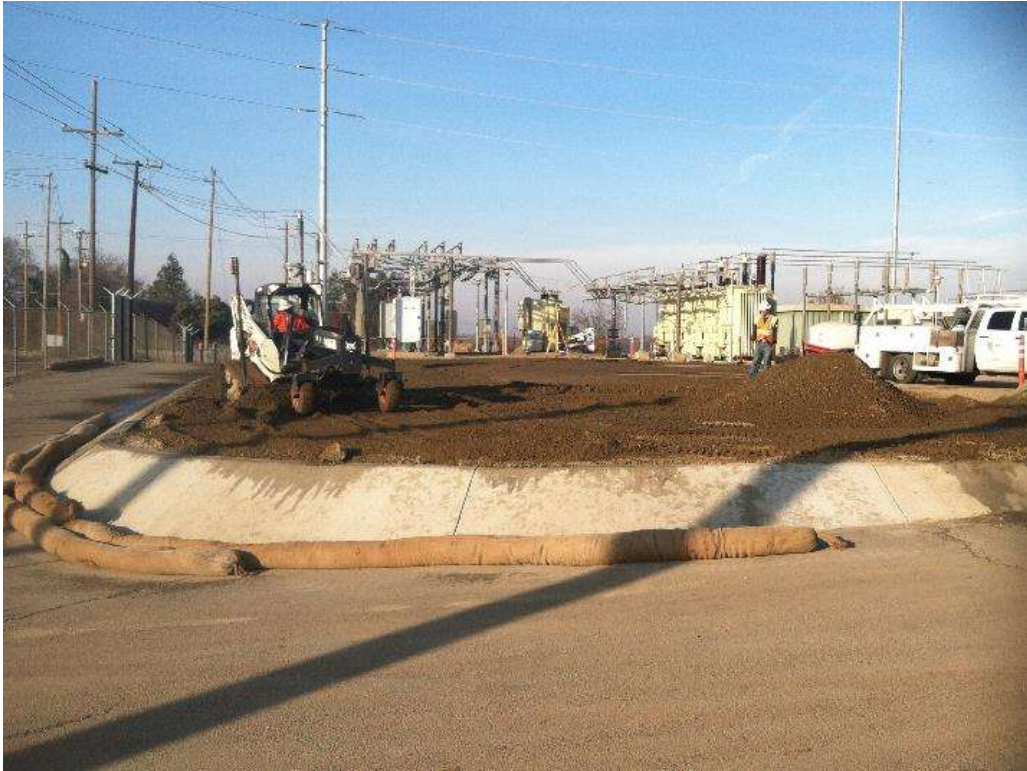
Figure 1 – Paving activities continued at the Cressey Substation during the subject period. View north, 12/17/15.
