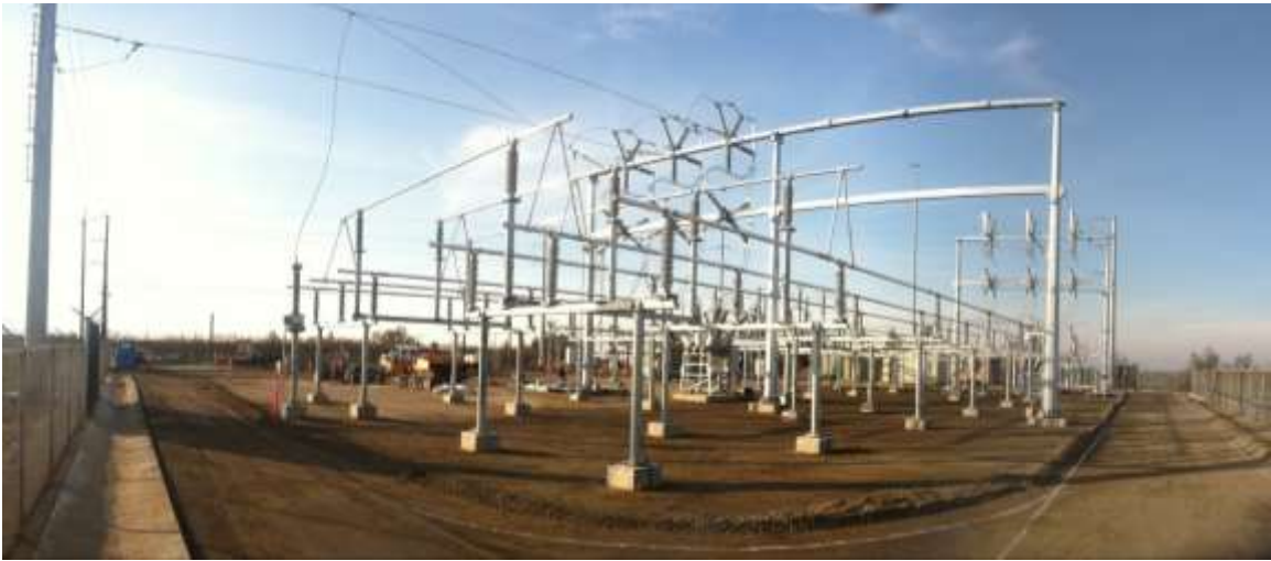
Figure 3 – Grading and paving work continued at Cressey Substation during the subject period. View northwest, 12/17/15.
