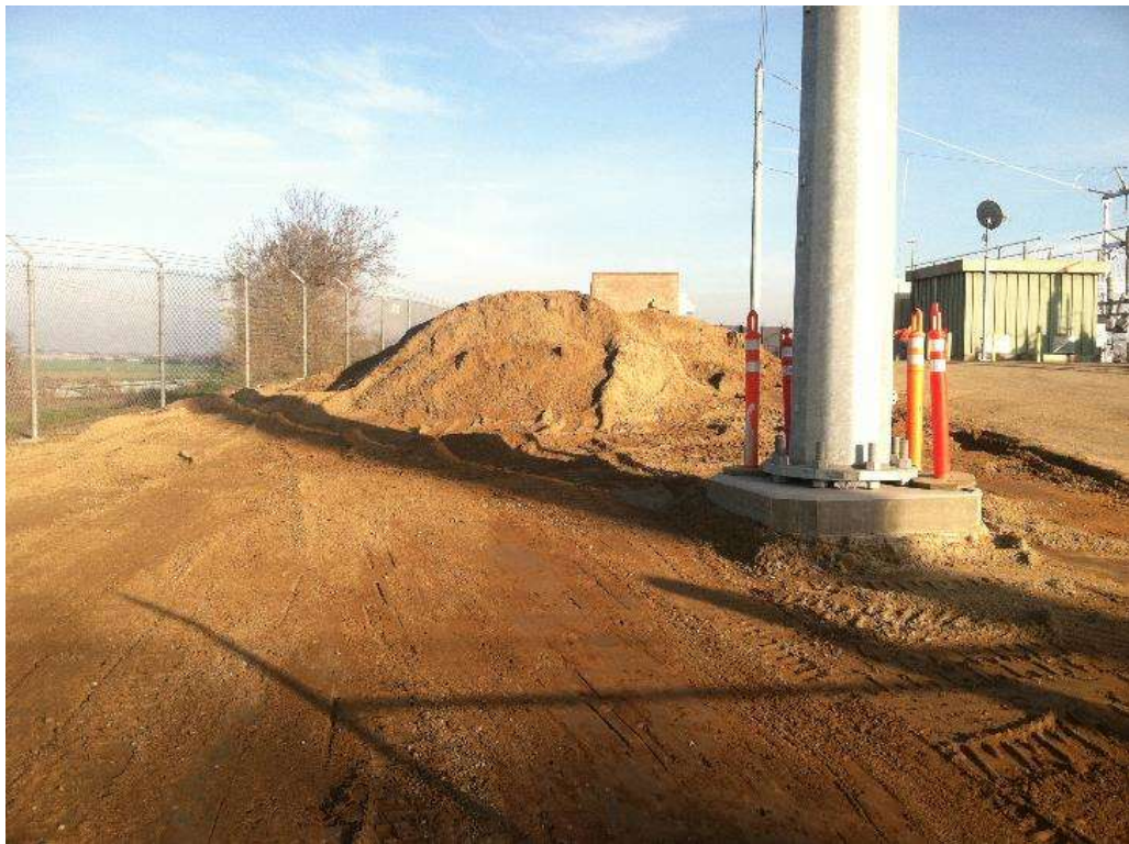
Figure 2 – Grading and paving work continued at Cressey Substation during the subject period. View east, 12/17/15.
