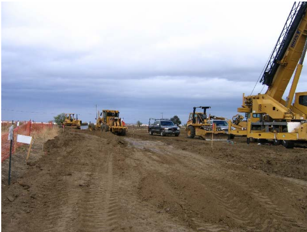
Figure 2 – Access road being graded and prepared on north side of Sand Creek, October 16, 2007.
