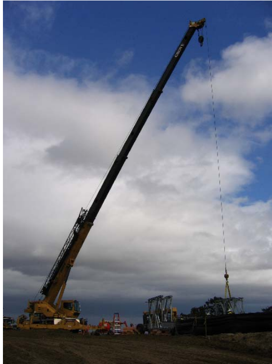
Figure 1 – Crane at staging yard on north side of Sand Creek moving bridge components for assembly, October 16, 2007.
