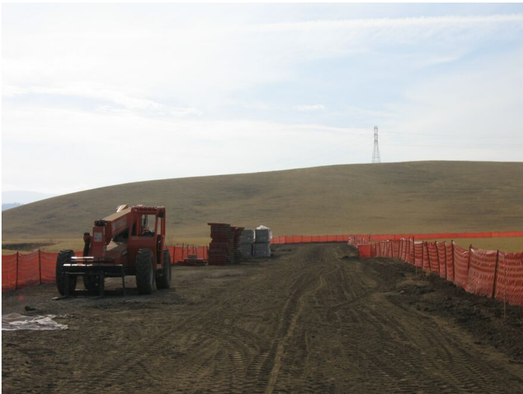
Figure 2 – Wildlife exclusion fencing installed along the access road to the substation, November 8, 2007.
