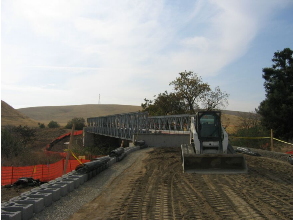
Figure 1 – Crews working on the keystone retaining wall on the north side of Sand Creek, November 8, 2007.
