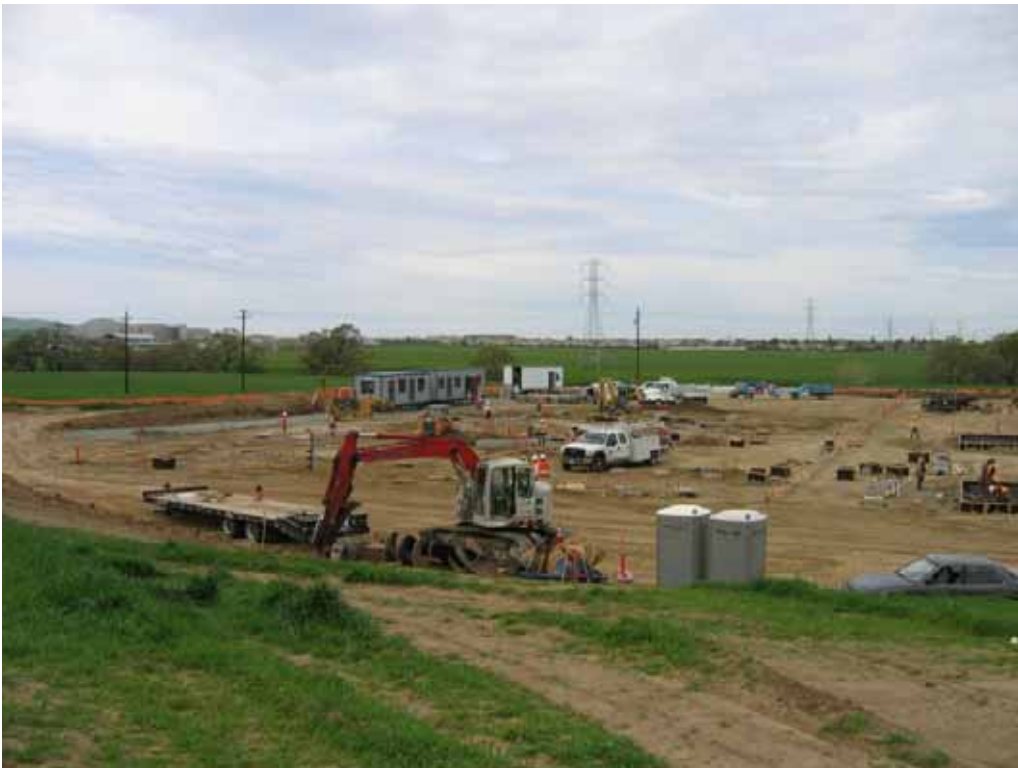
Figure 2 – View of substation site looking northwest, March 12, 2008.
