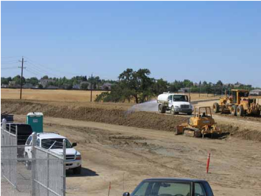
Figure 4 – Water truck watering earthen berm around substation, July 2, 2008.
