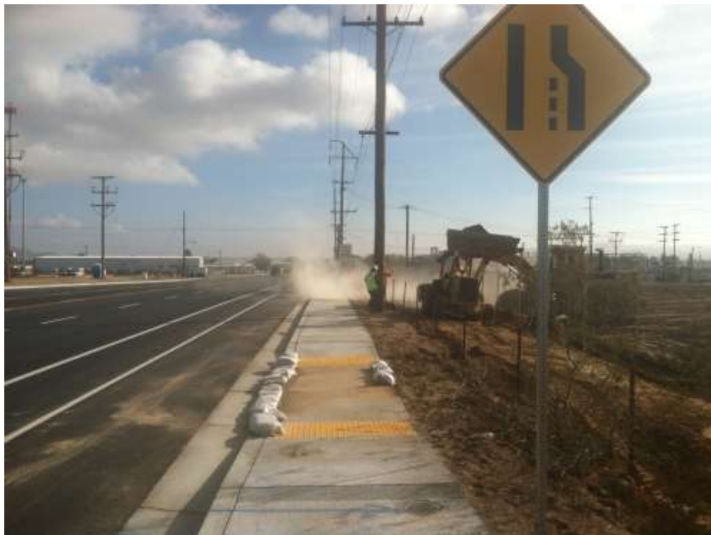
Figure 7 – Dust was observed leaving the Project site. The issue was swiftly corrected. View east, December 4, 2014.
