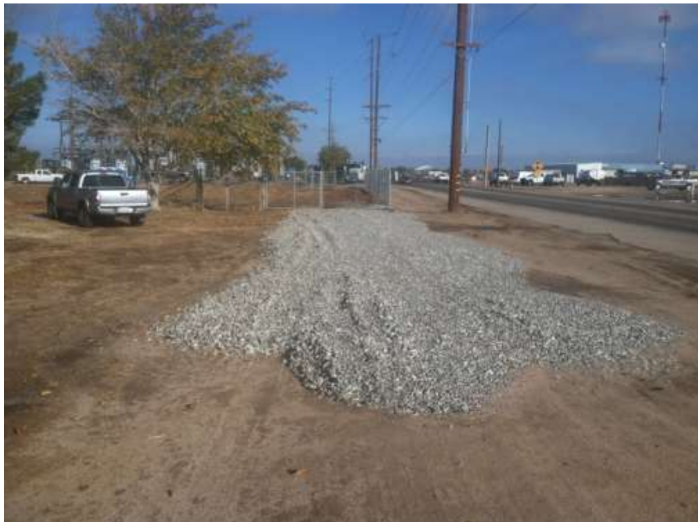
Figure 2 – Gravel apron and additional entrance was installed to accommodate longer vehicles delivering soil to the site. View north, December 4, 2014.
