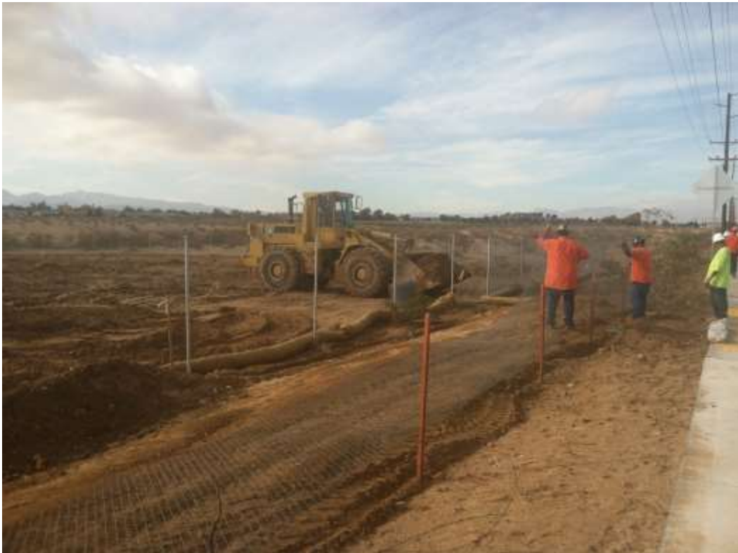
Figure 4 – Existing fencing, along northern work limits, was moved outward so that necessary grading could occur. View west, December 4, 2014.
