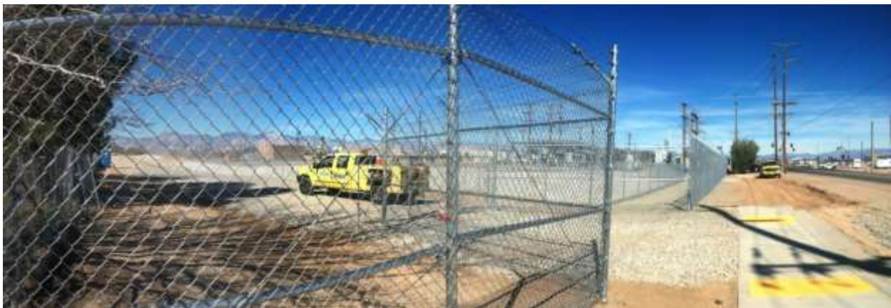
Figure 2 – Panoramic view of construction progress, from southeast corner of site. Fence installation occurred during the subject period. View northwest, 01/08/15 above, 02/06/15 middle, and 02/12/15 below.
