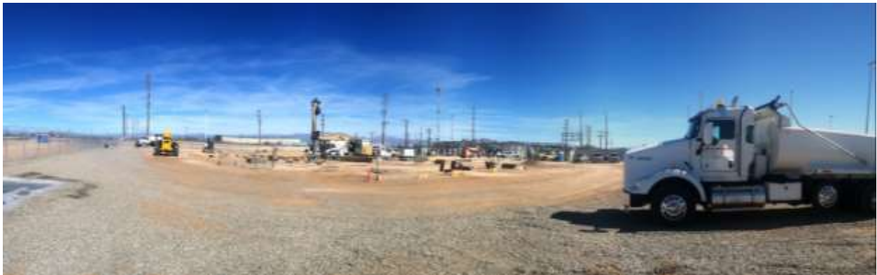
Figure 1 – Gravel and materials continue to be stored on the substation pad. View northeast, 01/27/15 above, 02/06/15 middle, 02/12/15 below.
