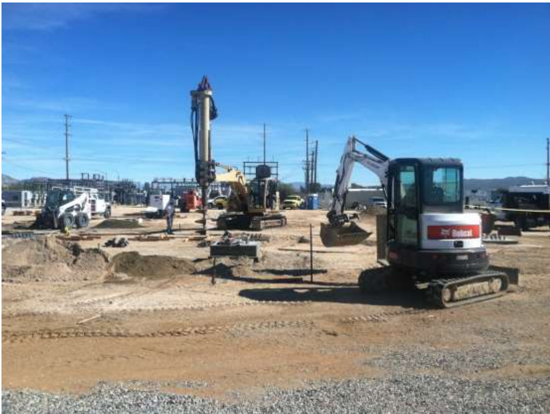
Figure 3 – Augering, trenching, and foundation installation continued in the substation expansion area. View northeast, 02/12/15.
