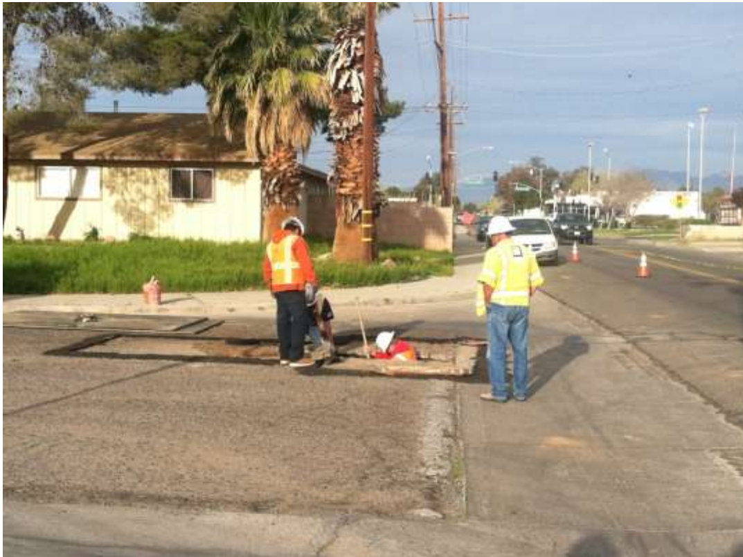
Figure 4 – Boring work for telecom lines continued during the subject period. View west, 03/17/15.
