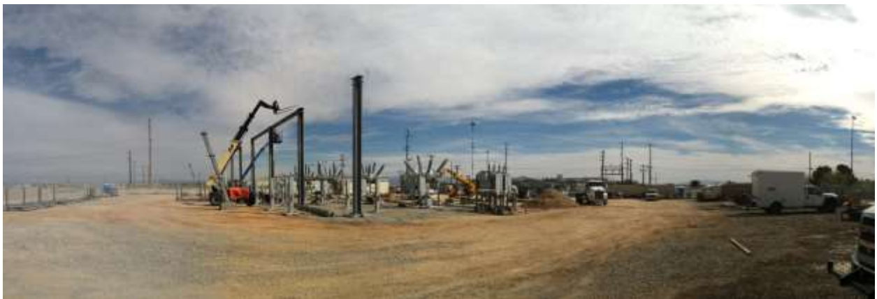
Figure 1 – Installation of the substation pad continued during the subject period. View northeast, 01/27/15 above, 02/06/15 middle, 03/17/15 below.
