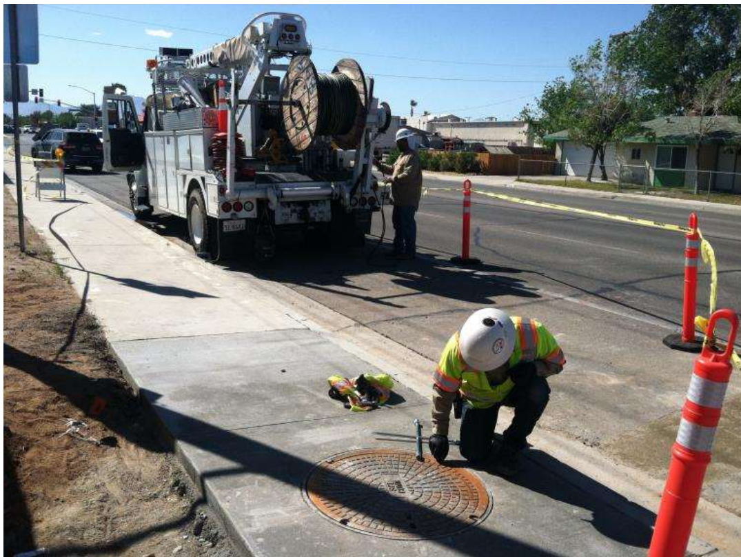
Figure 4 – Fiber optic work was completed at the SCE Ridgecrest Service Center during the subject period. View northwest, 04/13/15.
