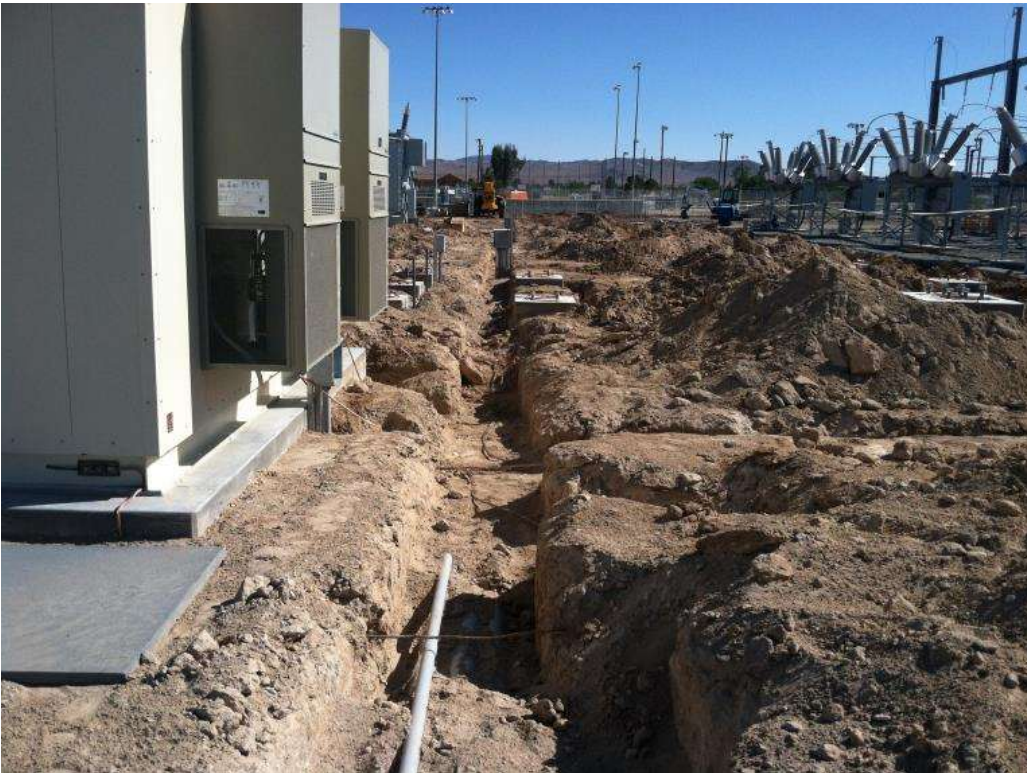
Figure 2 – Underground conduit installation occurred within the Substation expansion area during the subject period. View south, 04/13/15.
