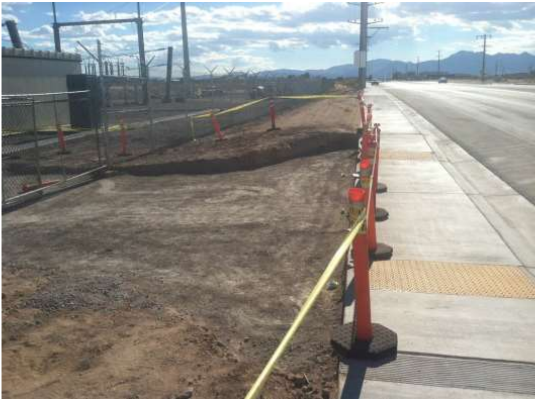
Figure 3 – Installation of a driveway apron began during the subject period. View west, 6/11/15.
