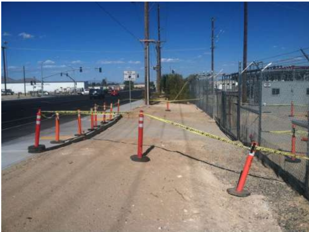
Figure 2 – Installation of a driveway apron began during the subject period. View east, 6/11/15.
