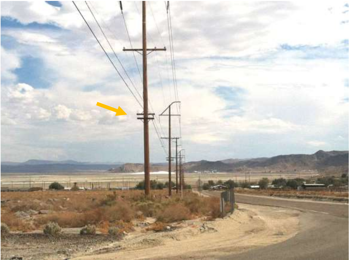
Figure 3 – Recently installed cable and arms along telecom route between McGen and Searles Substations. View south, 7/30/2015.
