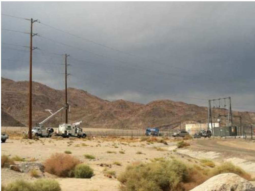
Figure 2 – Line crews installed telecom cables between McGen Substation (pictured) and Searles Substation during the subject period. View northeast, 7/30/2015.
