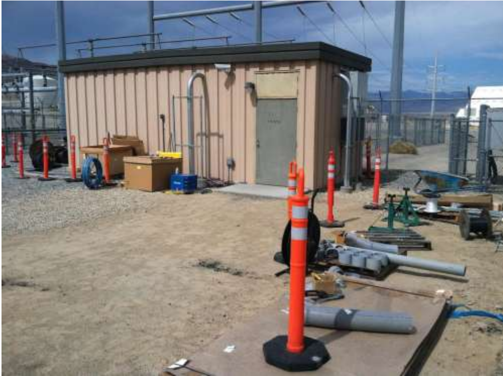
Figure 1 – Electrical work continued at McGen Substation inside the MEER building during the subject period. View northeast, 7/30/2015.
