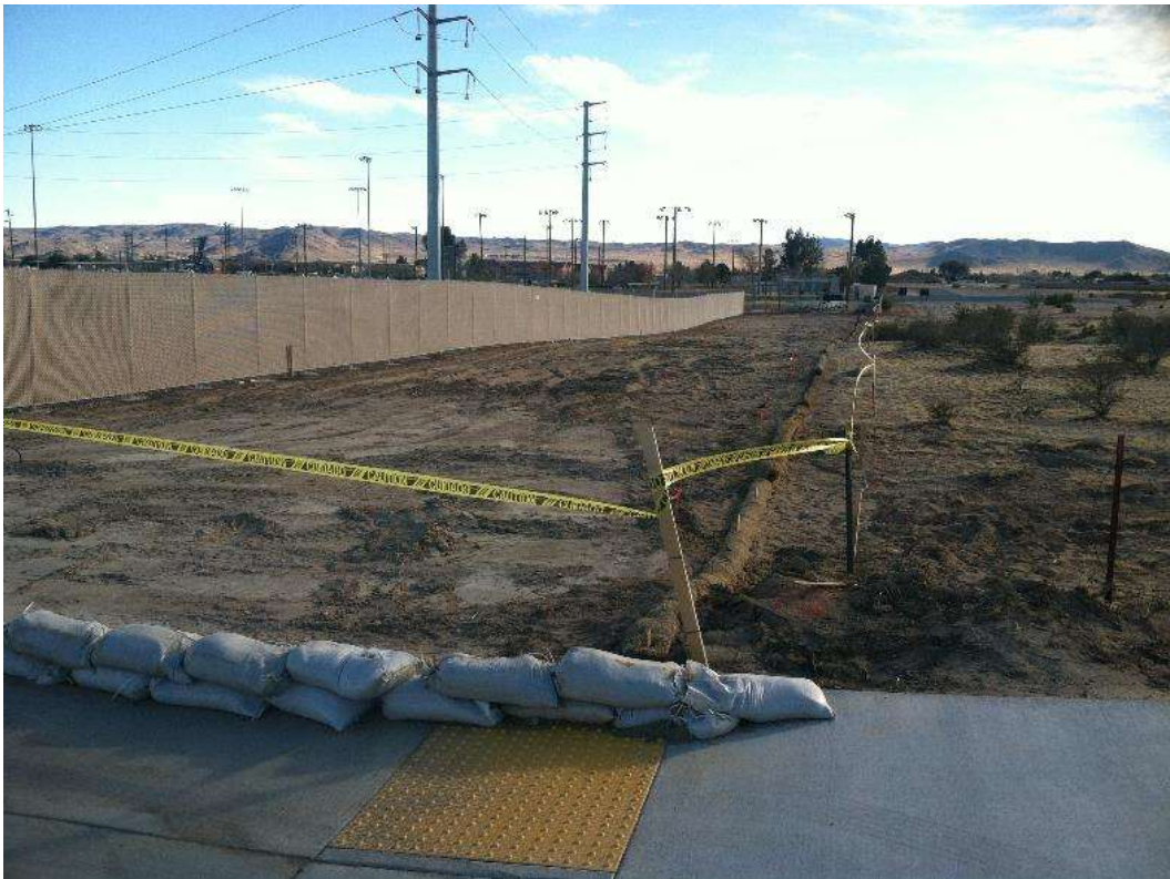
Figure 3 – SWPPP BMPS were in place along the edges of work areas. View southeast (12/11/15).
