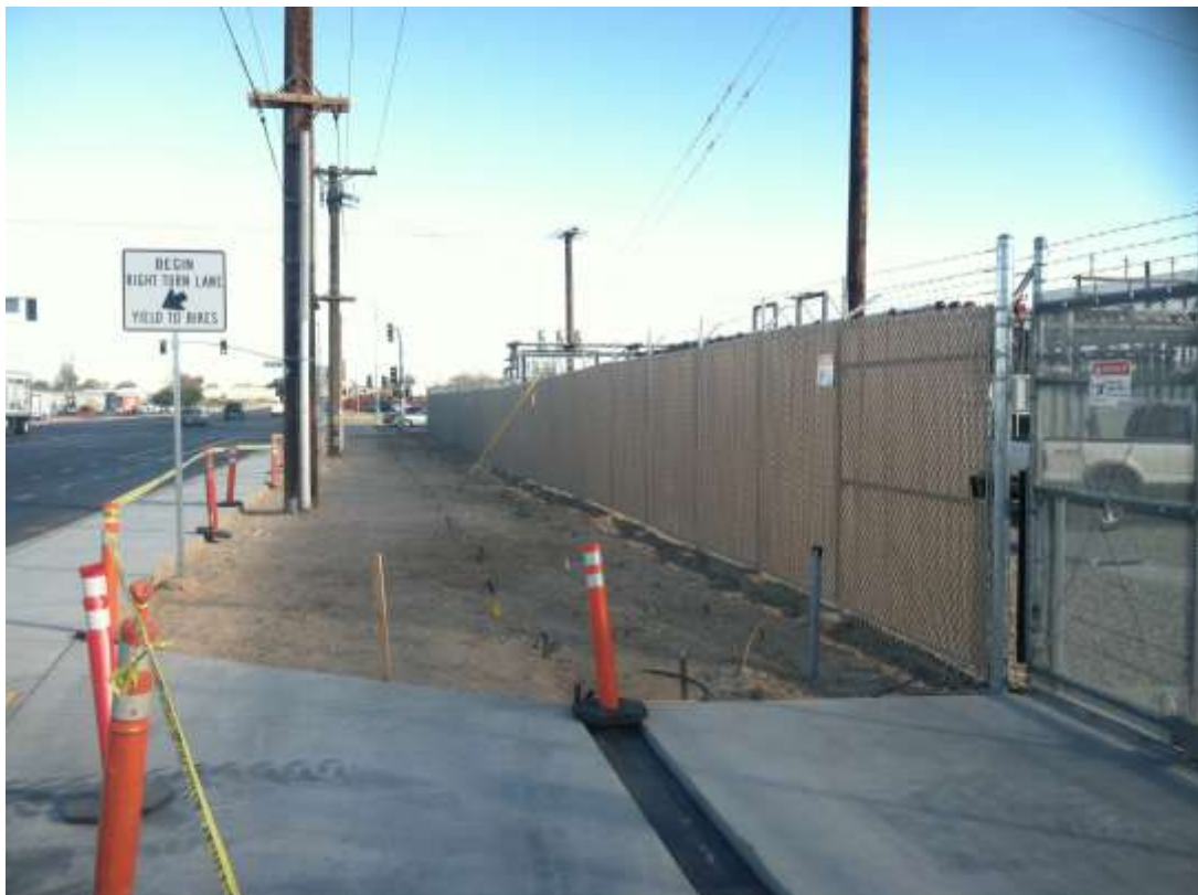
Figure 1 – Landscape crews installed irrigation lines along the northern edge of the substation during the subject period. View east (12/3/15 above, 12/11/15 below).
