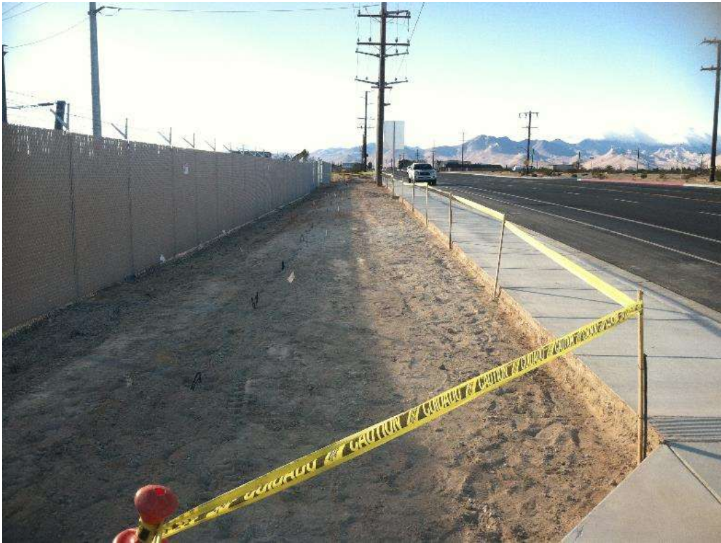
Figure 2 – Landscape crews installed irrigation lines along the northern edge of the substation during the subject period. View west (12/11/15).
