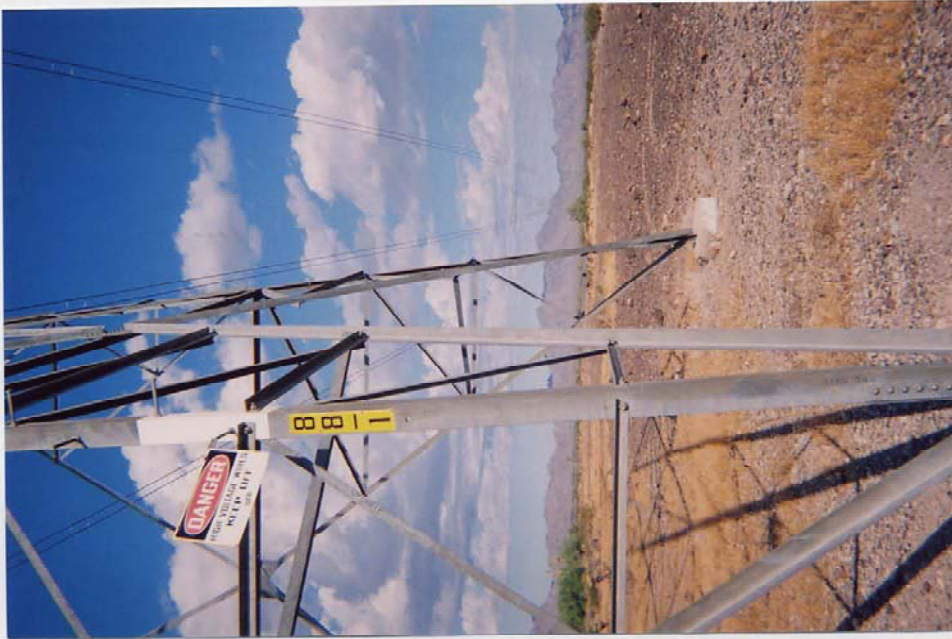
(No. 1593) 8-3-2006 - DPV1 Tower is numbered No. 88-1; the tower is located east of the Crystal Mtn. Rd. approaching the Kofa Nat'l Wildlife Refuge, Az. 8703 20060903
