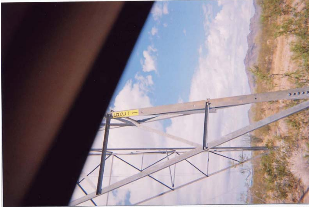
8-3-2006 - DPV1 Tower No. 62-1 is the first DPV1 tower outside the eastern boundary of the Kofa Nat'l Wildlife Refuge on the left side (north) driving Pipeline Rd. east.
