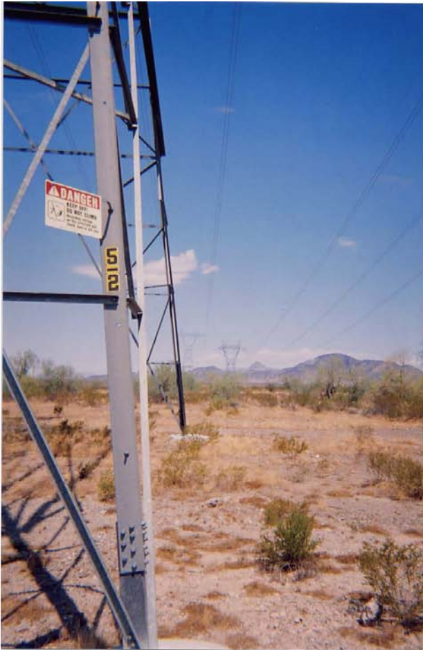
8-3-2006 - Harquahala-Hassayampa 500kV Line Tower No. 5-2 adjacent to DPV1 Tower No. 14-1 Tower off Salome Hwy. in Harquahala Vly., Az.
