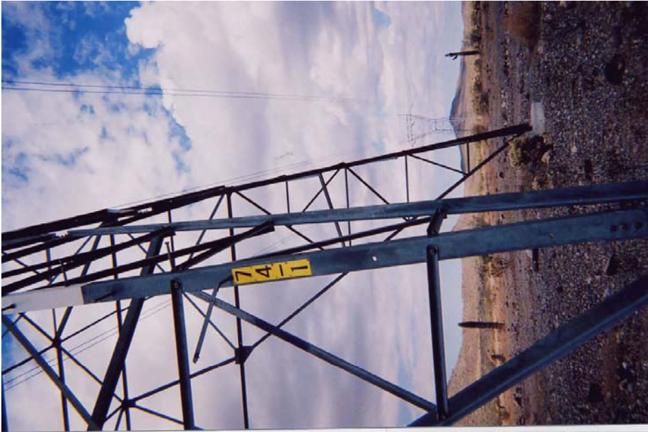
8-3-2006 - DPV1 Tower No. 74-1 on the northerly side of Pipeline Rd. in the Kofa Nat'l Wildlife Refuge, Az. looking toward Tower No. 74-2 southerly of the road.
