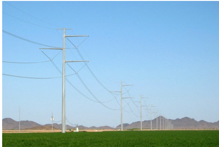
Photo 1 - 500 kV Tubular steel poles east from Harquahala
