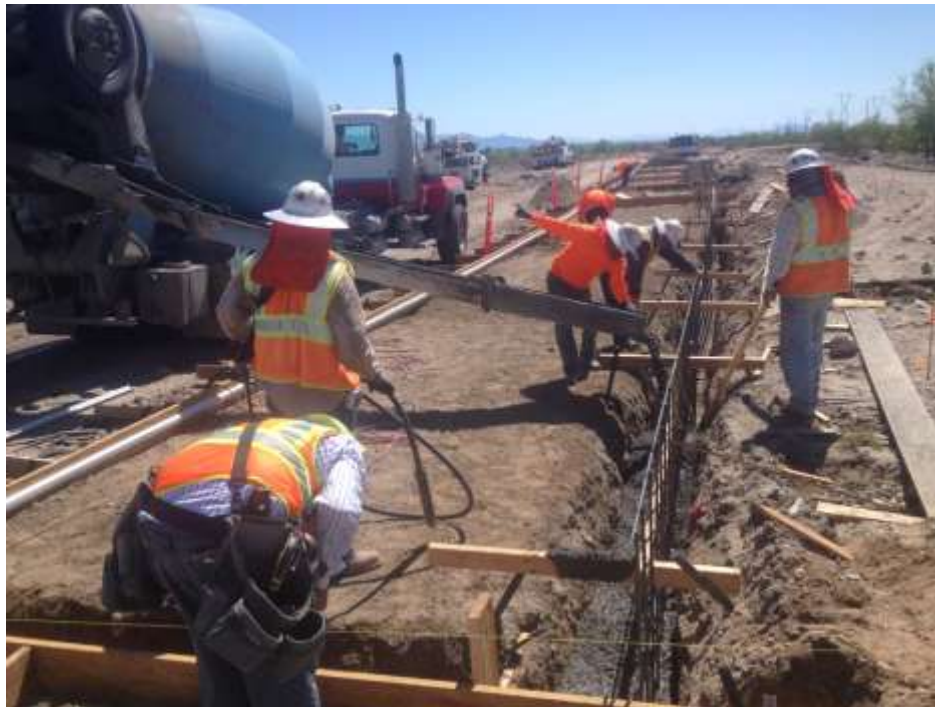
Figure 3. Concrete pouring for Arizona crossing along access road (Photo courtesy of FRED).
