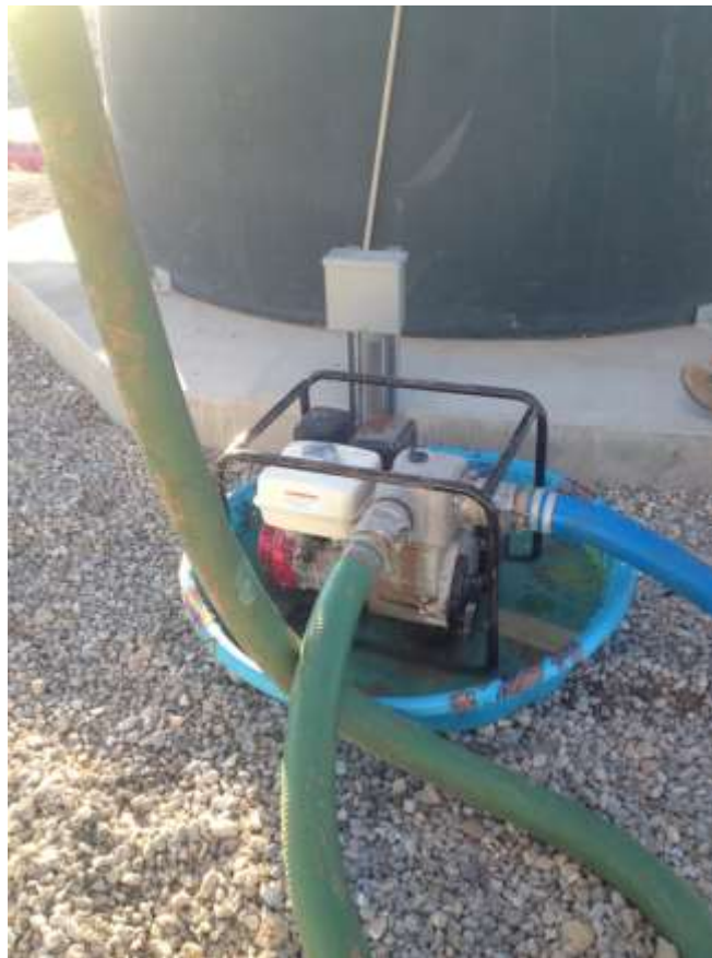
Figure 4. Pooled contaminated water near water tank in staging area (Photo courtesy of FRED).
