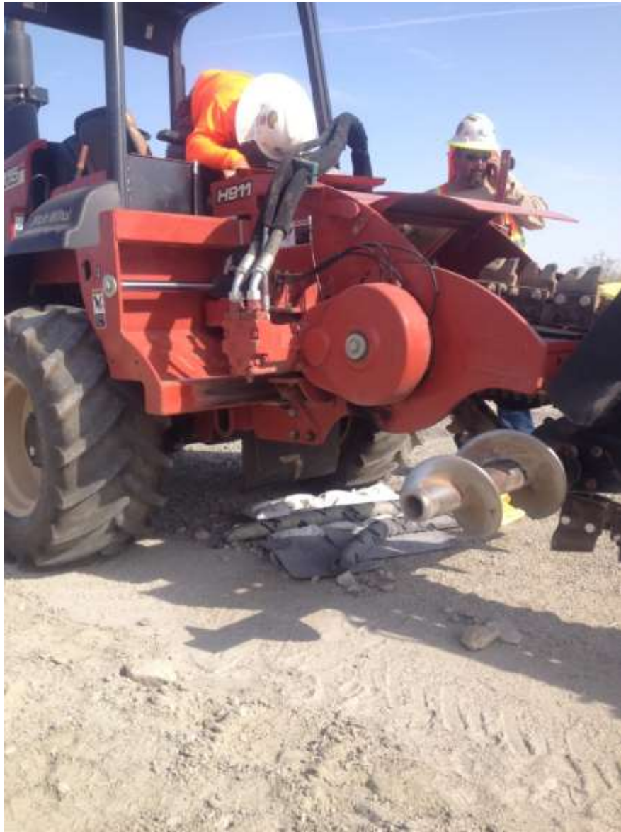
Figure 5. Hydraulic leak from excavator being contained by crew (Photo courtesy of FRED).
