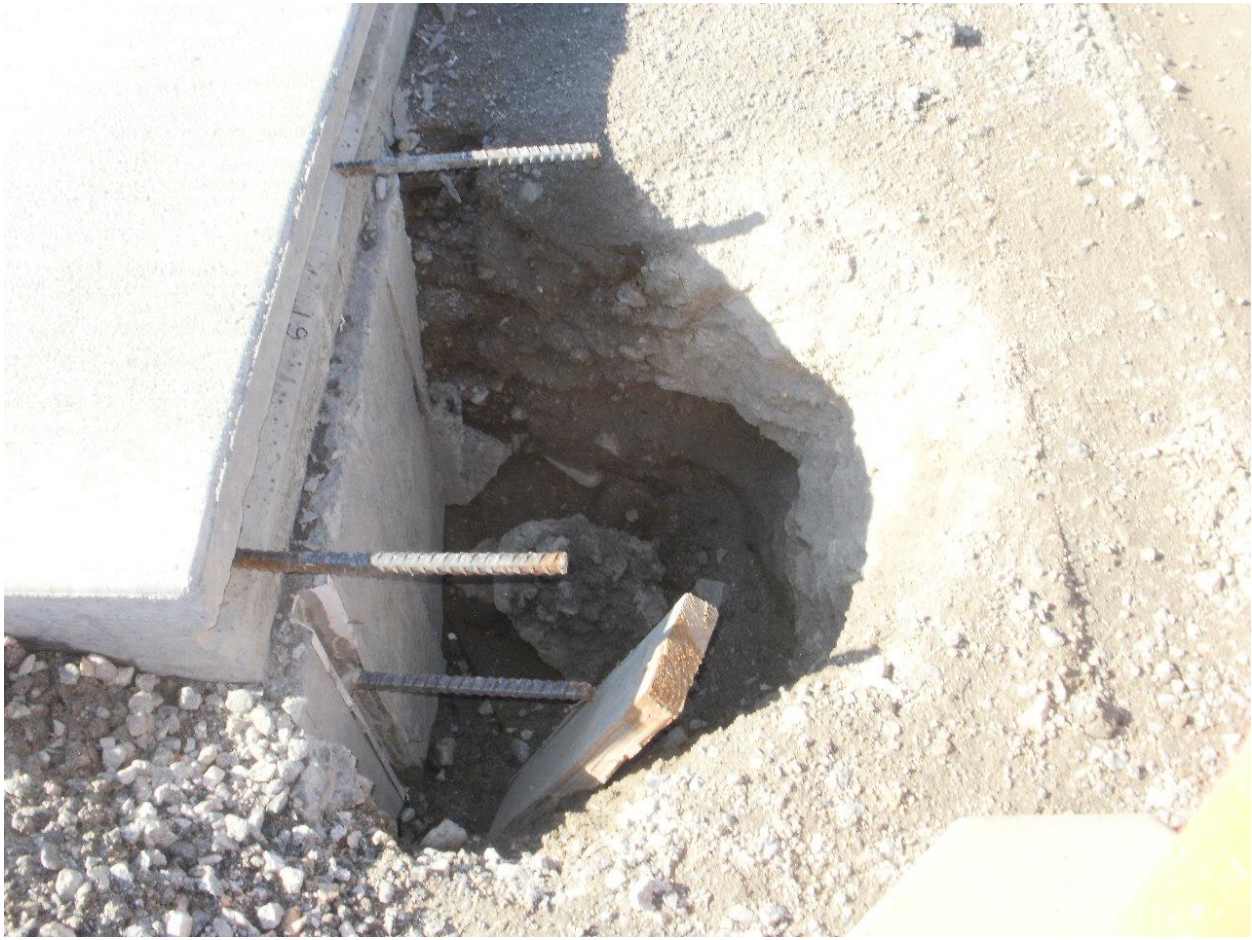
Figure 5. Footer hole with wildlife ramp eroded away. On-site monitors will assess and ensure that crews repair any eroded ramps.
