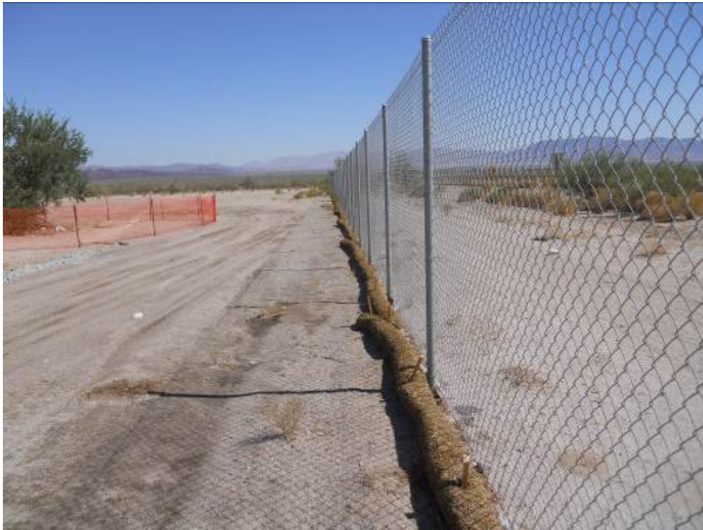
Figure 3: Straw wattles installed along existing eastern chain link fence line at DC1.
