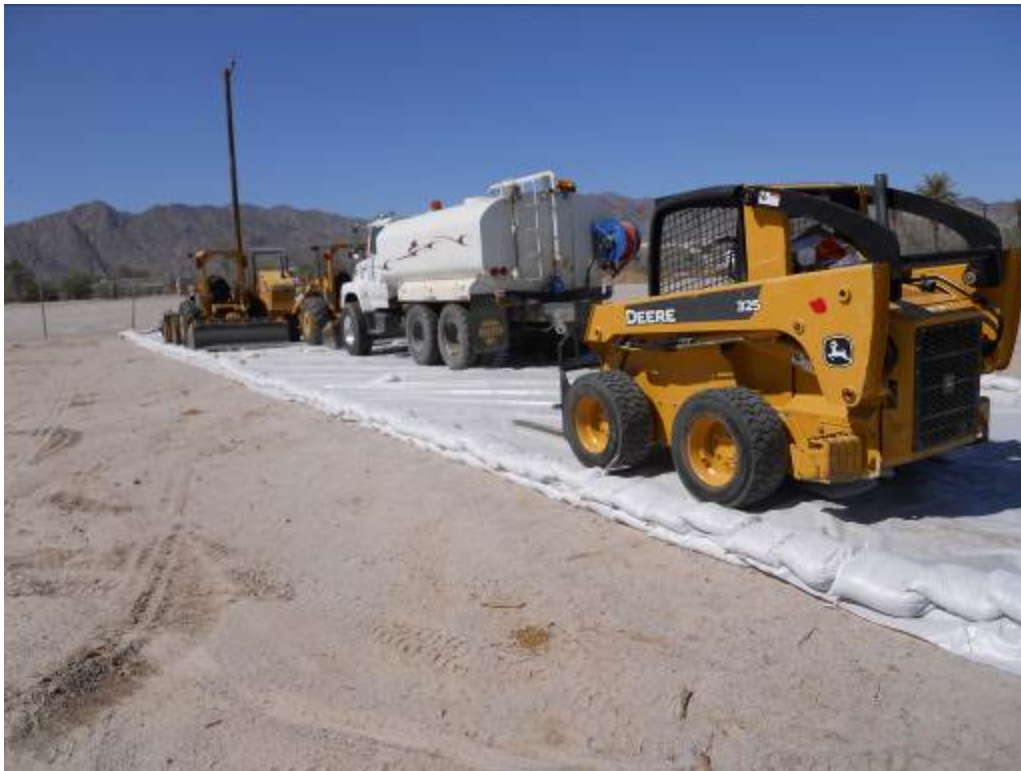
Figure 5: Plastic sheeting with sandbag anchors installed for heavy equipment overnight parking at DC1.
