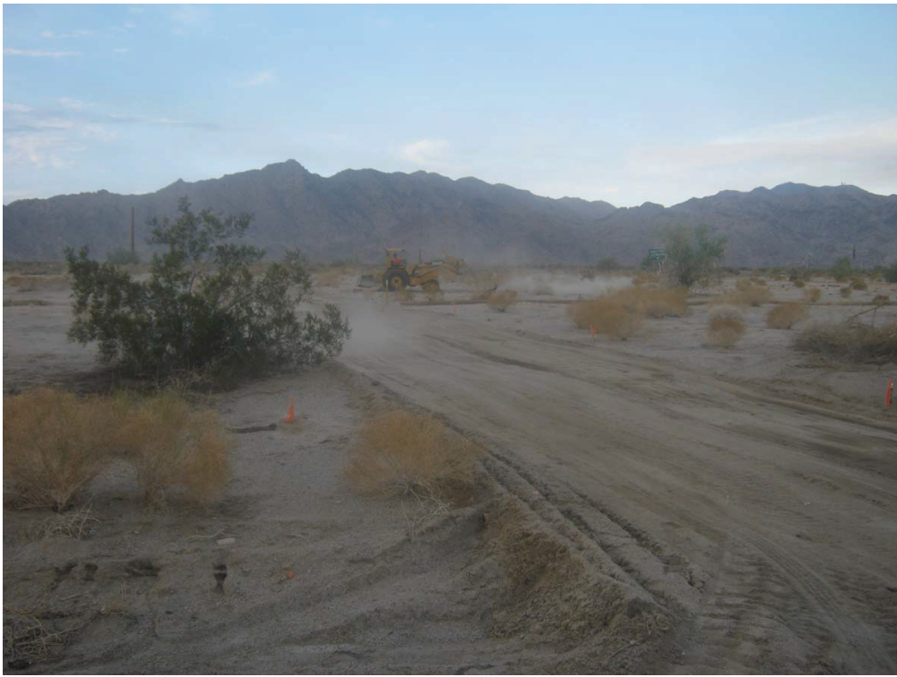
Figure 5: Excessive dust during soil removal activities as DC2.
