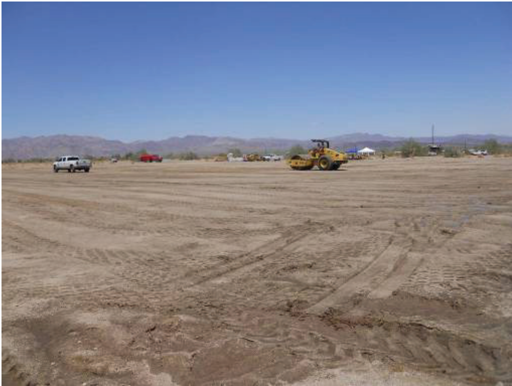
Figure 3: Ongoing grading activities occurring at DC2 Yard. View southwest from northeast corner of yard.
