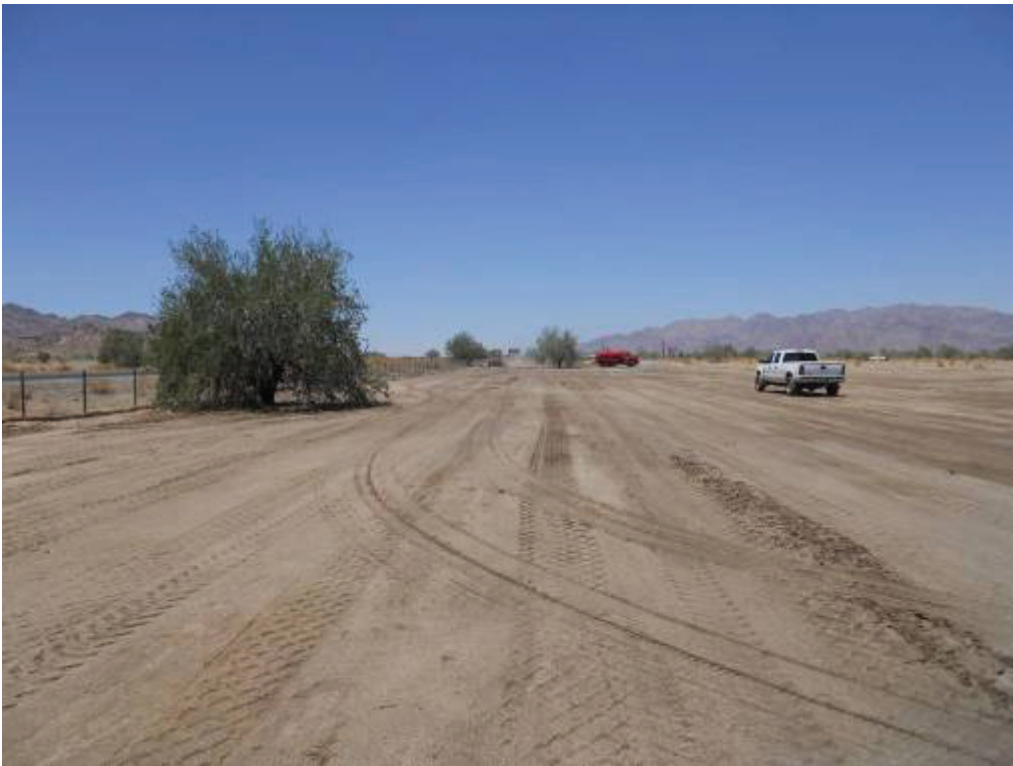
Figure 2: Ongoing construction activities occurring at DC2 Yard. View west along southern boundary of yard.
