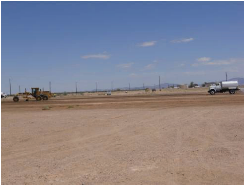
Figure 5: Dust suppression being provided via water truck during grading activities at Blythe Construction Yard.
