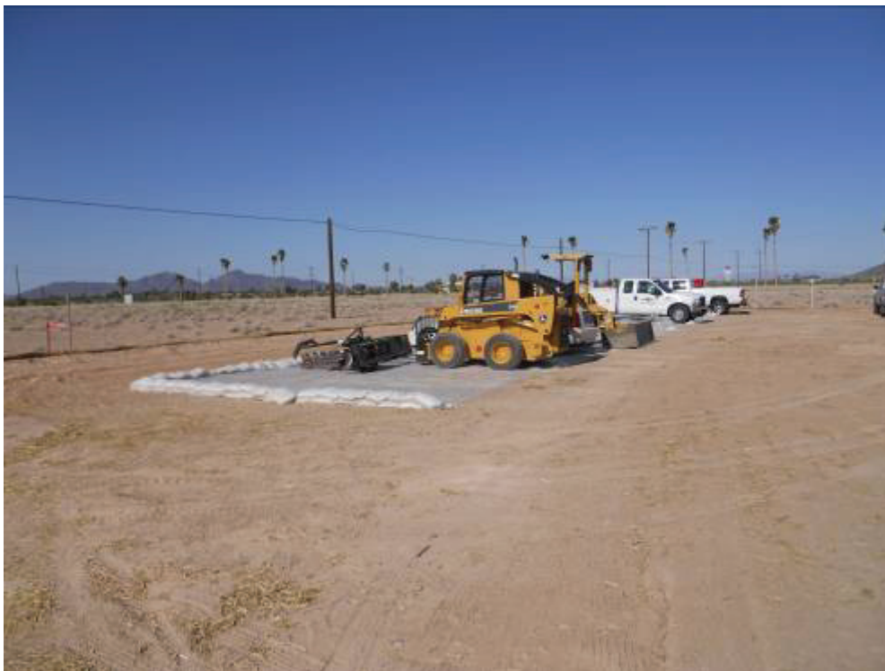
Figure 6: Plastic sheeting underneath overnight parking/storage area at Blythe Construction Yard.
