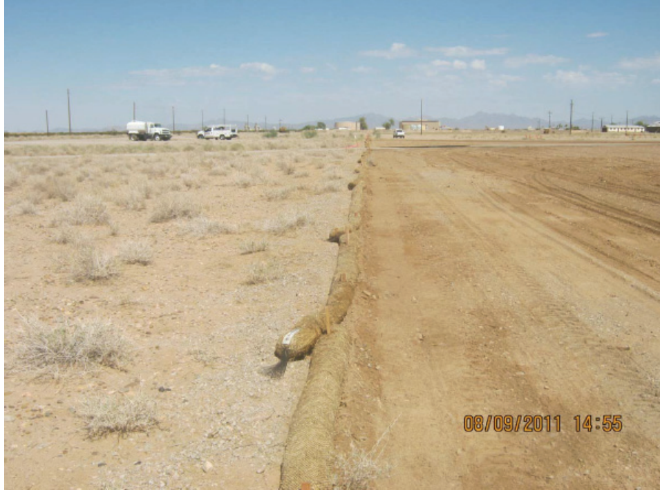
Figure 1: BMPs (straw wattles) were installed around the perimeter of the Blythe Construction Yard.
