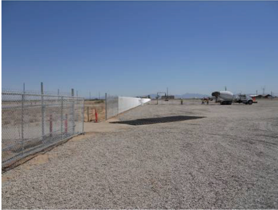
Figure 1: Ongoing activities at the Blythe Construction Yard included installation of fence posts.
