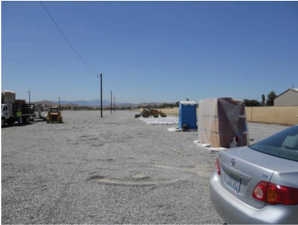
Figure 5: Activities at the Menifee Construction Yard included removal of straw wattles and heavy equipment.
