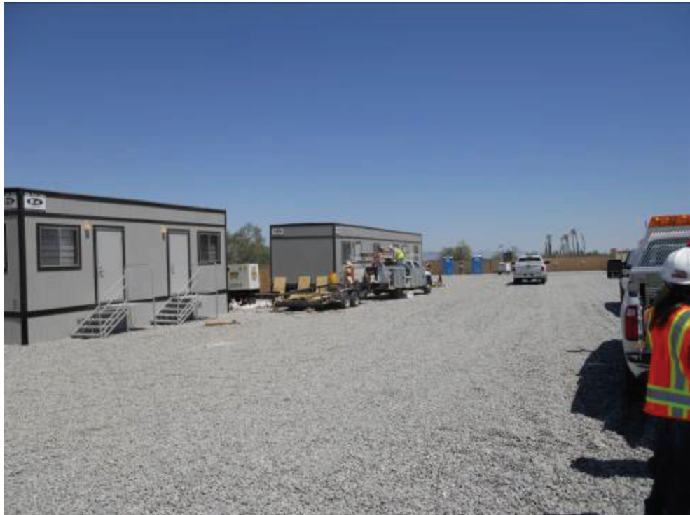
Figure 4: Office trailers have been delivered at DC2 Construction Yard. Crews were observed installing skirting.
