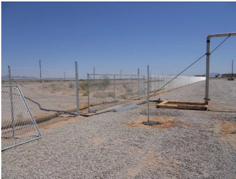
Figure 2: New gate installed along the northern fence boundary of the Blythe Construction Yard.
