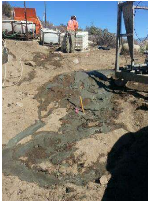
Figure 5. Grout spill at Tower 1045.
