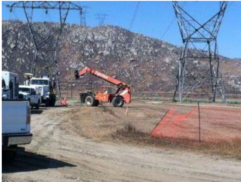
Figure 3. Forklift driving outside of the disturbance area on the access road to Tower 1122.
