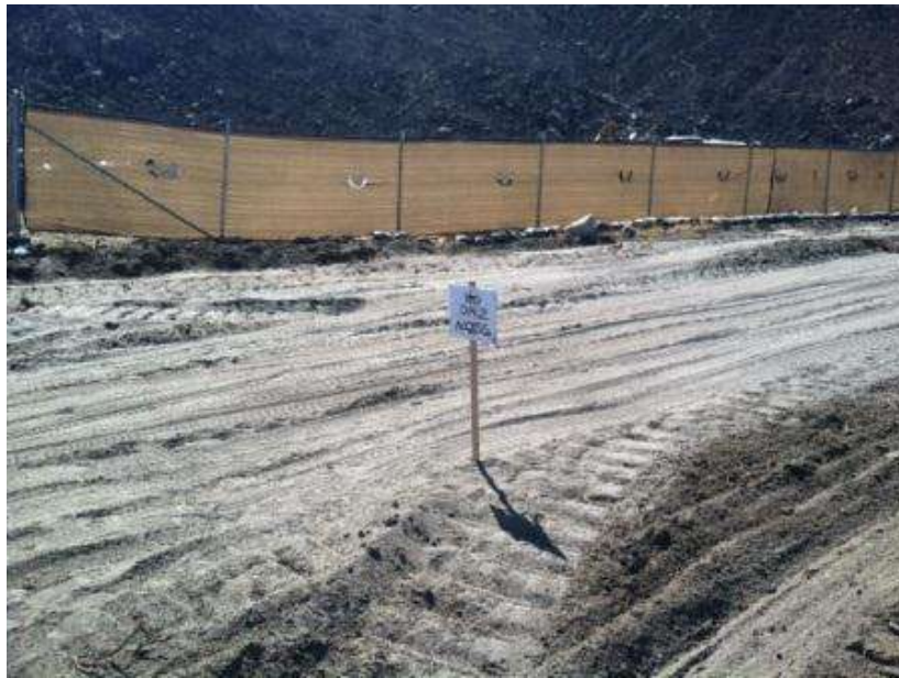
Figure 5. Delineation staking at HLZ H2 to prevent the use of the cleared firebreak areas that are not part of the approved project disturbance limits.
