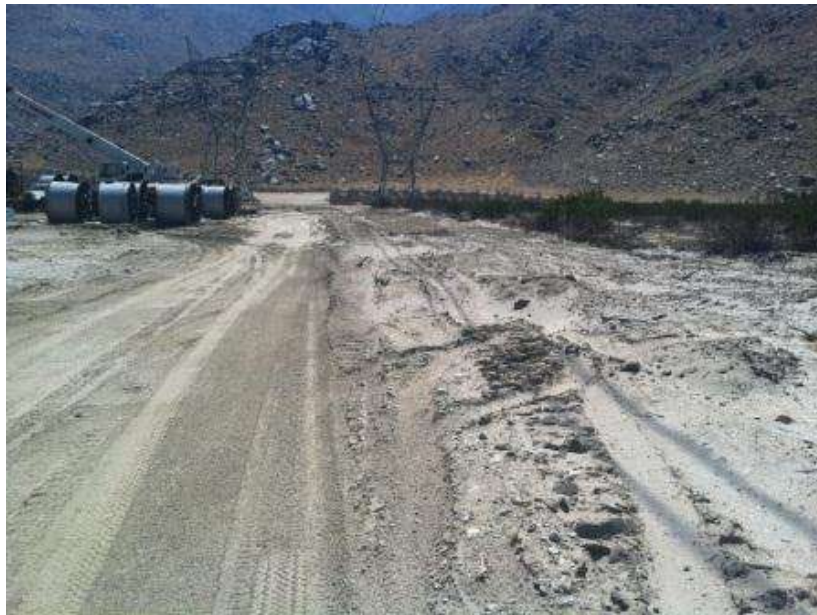
Figure 4. Vegetation cleared as a firebreak for the protection of construction equipment and materials at Wire Site 10 during the Silver Fire. (Area cleared is on the right side of the photo)
