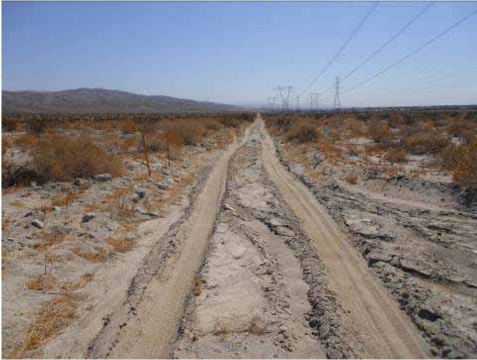
Figure 1: Access road within the Coachella Valley Preserve that was rejected by the CPUC EM under a TEWS request for parking due to the presence of potential habitat for Coachella Valley fringe-toed lizard.
