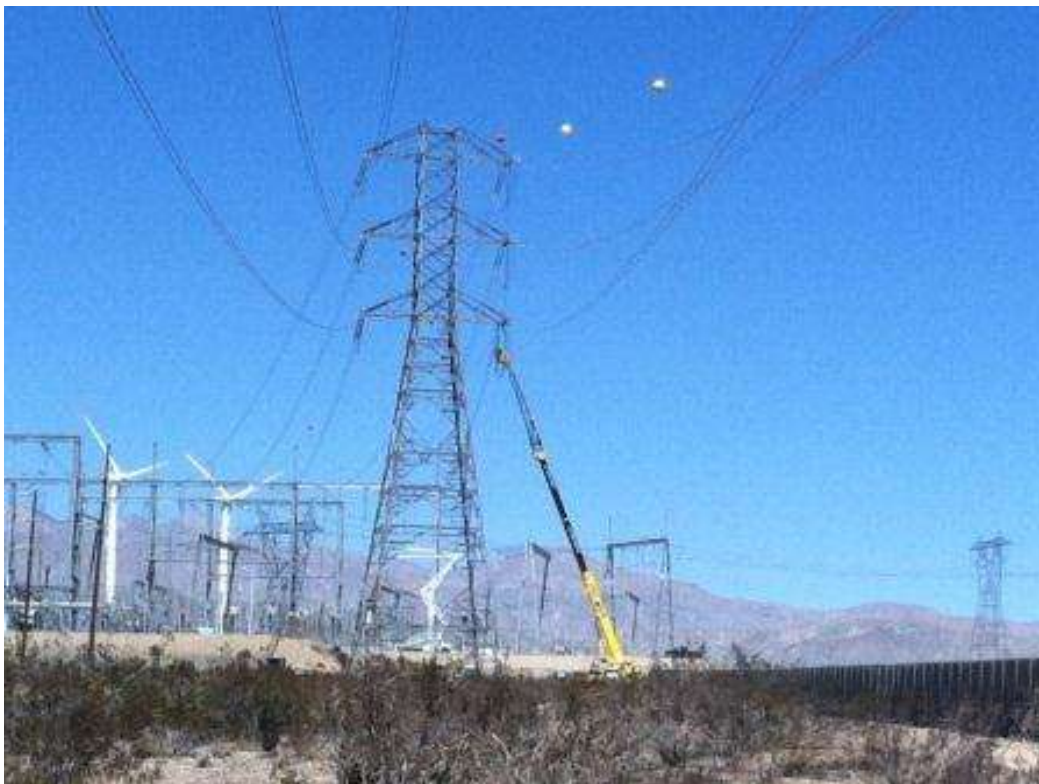
Figure 2. Wire stringing activities associated with rephrasing the conductor at Tower 1001 and the Devers Substation.
