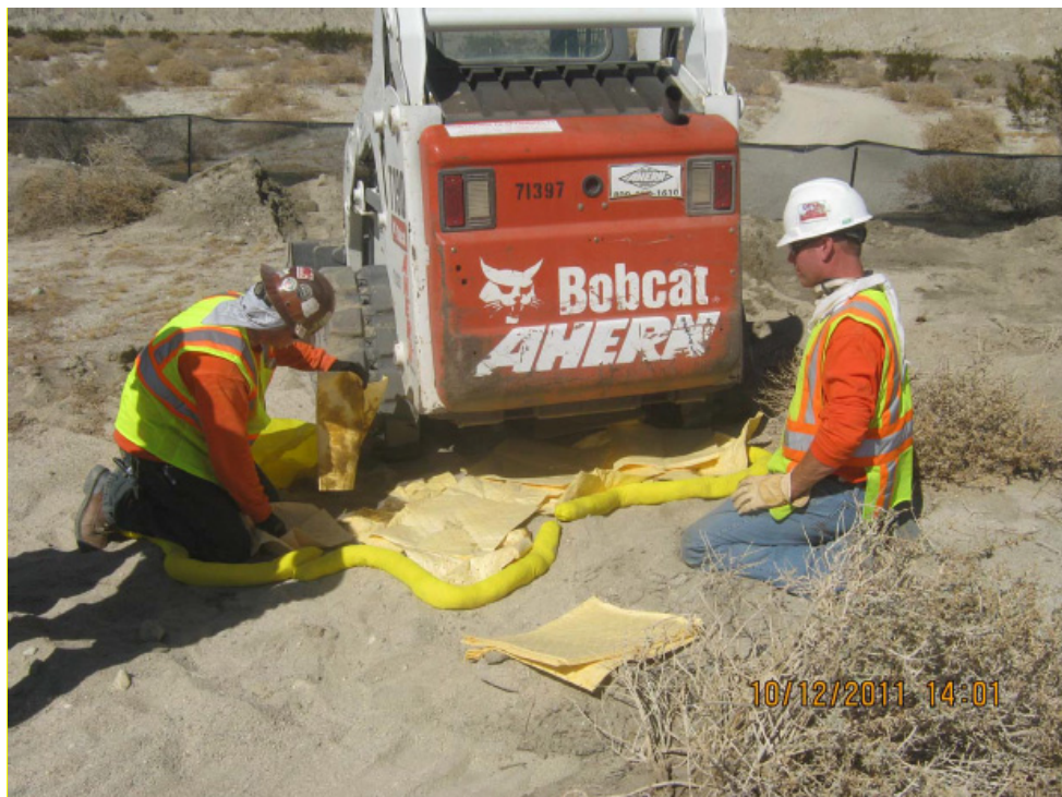
Figure 3: Small hydraulic fluid spill being contained during exclusionary fence installation at Tower #2132.
