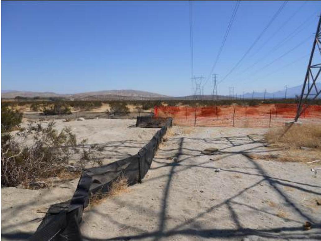
Figure 2: Exclusionary fencing has been installed at a tower location. Note avoidance of ESA (orange construction fencing).
