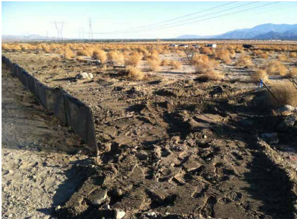
Figure 3: View southeast along partially completed fencing at Tower #2204. No open trenches were left overnight.
