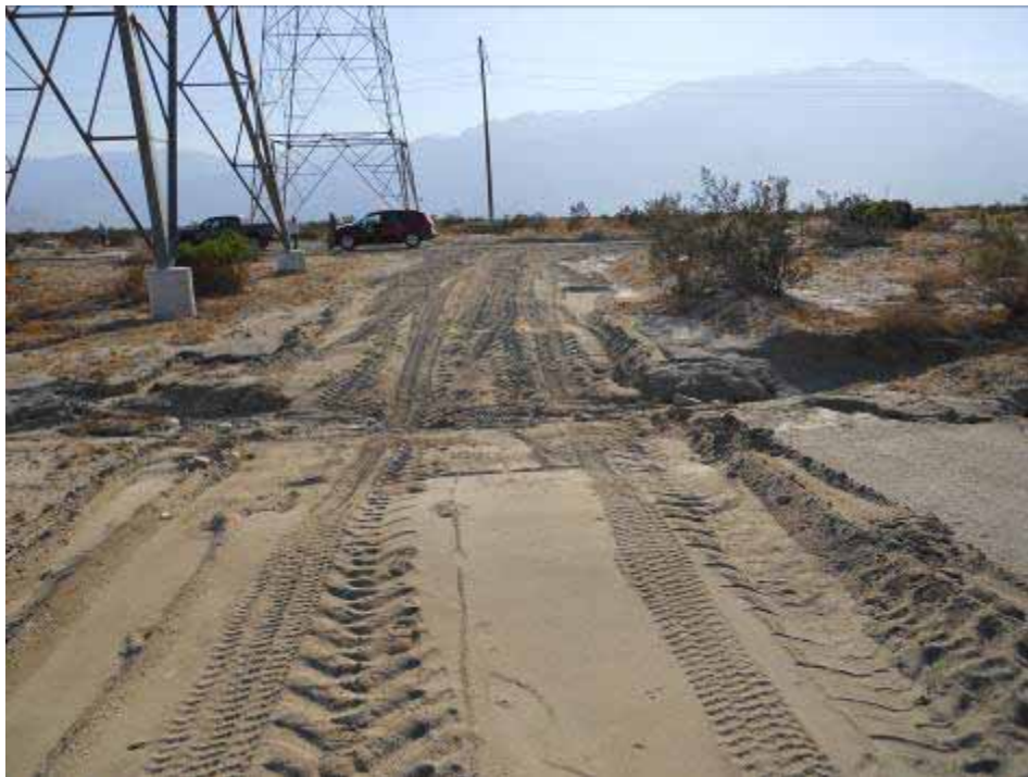
Figure 4: View south along stub road and across potential jurisdictional drainage at Tower #2101. Note fresh equipment tracks crossing drainage that were later confirmed to be the result of O&M crew in the area.
