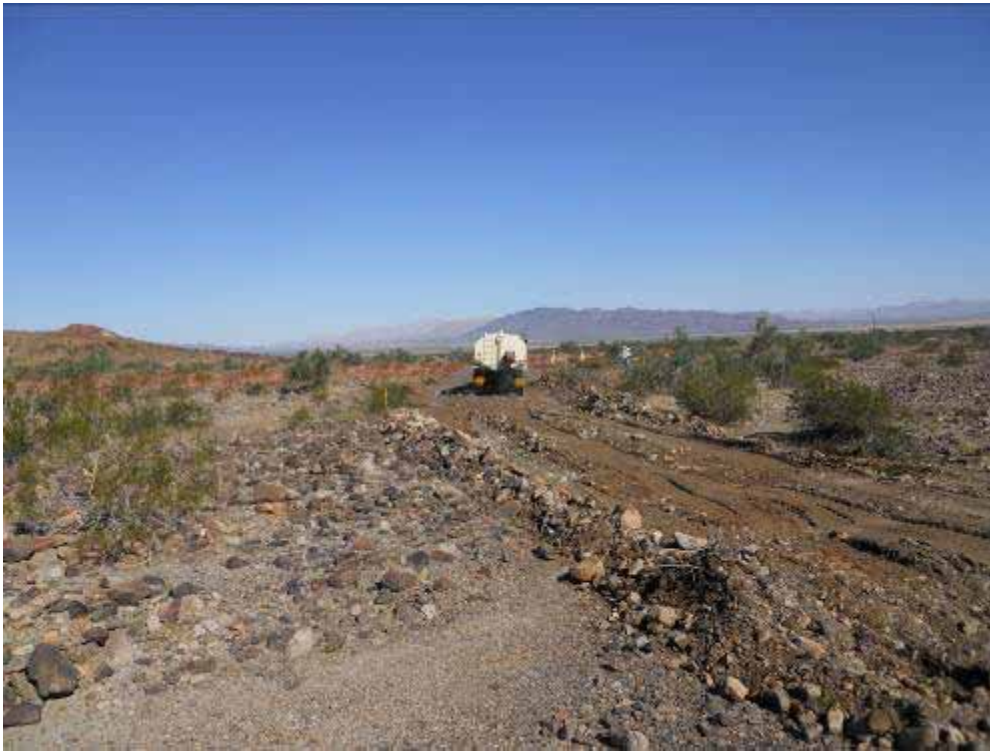
Figure 7: Rough grading of eastern access road and dust suppression occurring at Red Bluff Substation site.
