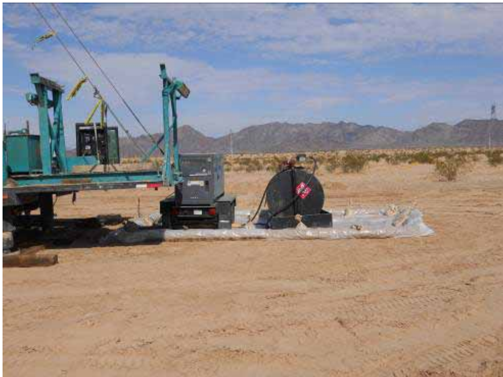
Figure 6: Secondary containment confirmed by CPUC EM at CRS. Note plastic sheeting and sandbag containment of generator and fuel tank.
