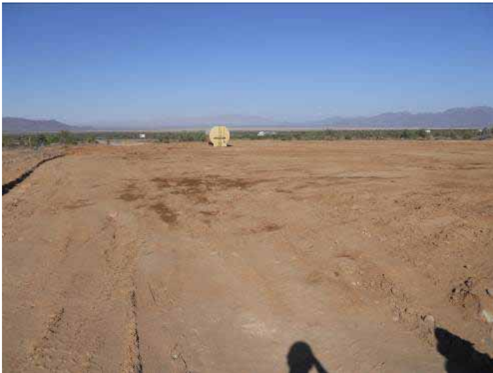
Figure 10: Area cleared and graded at Red Bluff site to accommodate well drilling activities.
