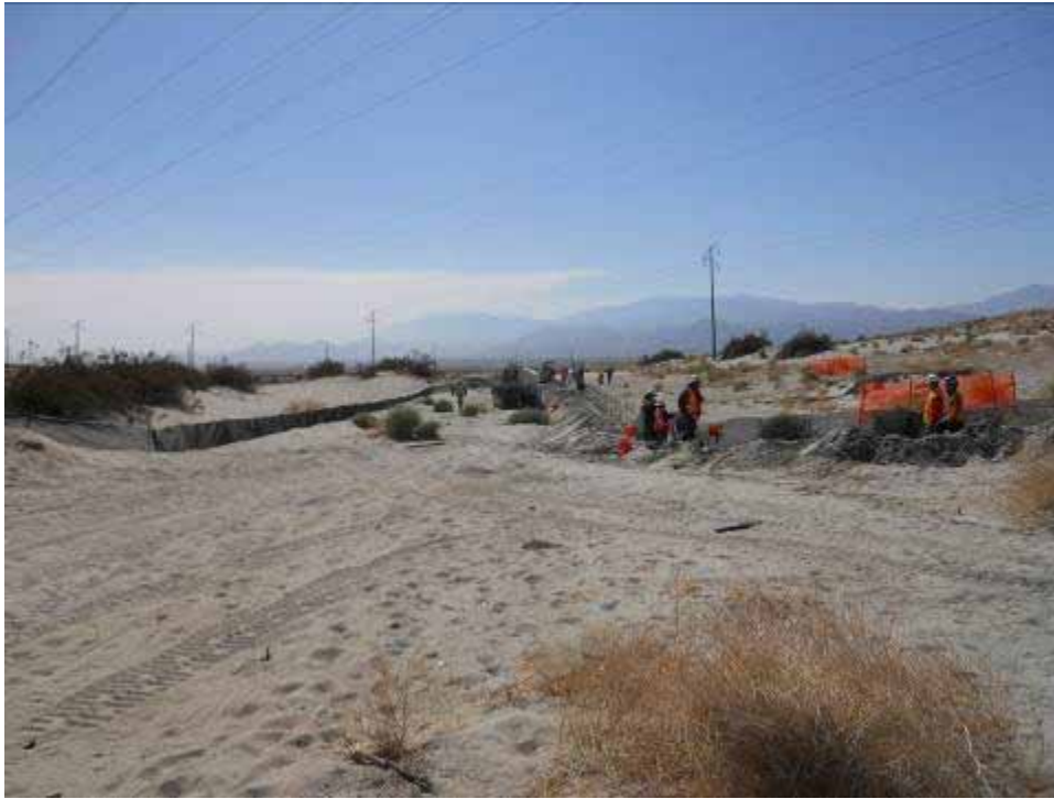
Figure 1: Exclusionary fence activities being conducted at Tower #2110. Note avoidance of ESAs marked with orange fencing.
