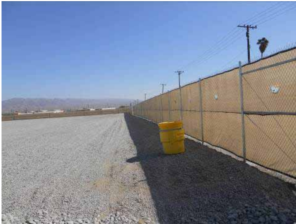
Figure 2: Activities at the Indio Construction Yard included fence installation and gravel placement.
