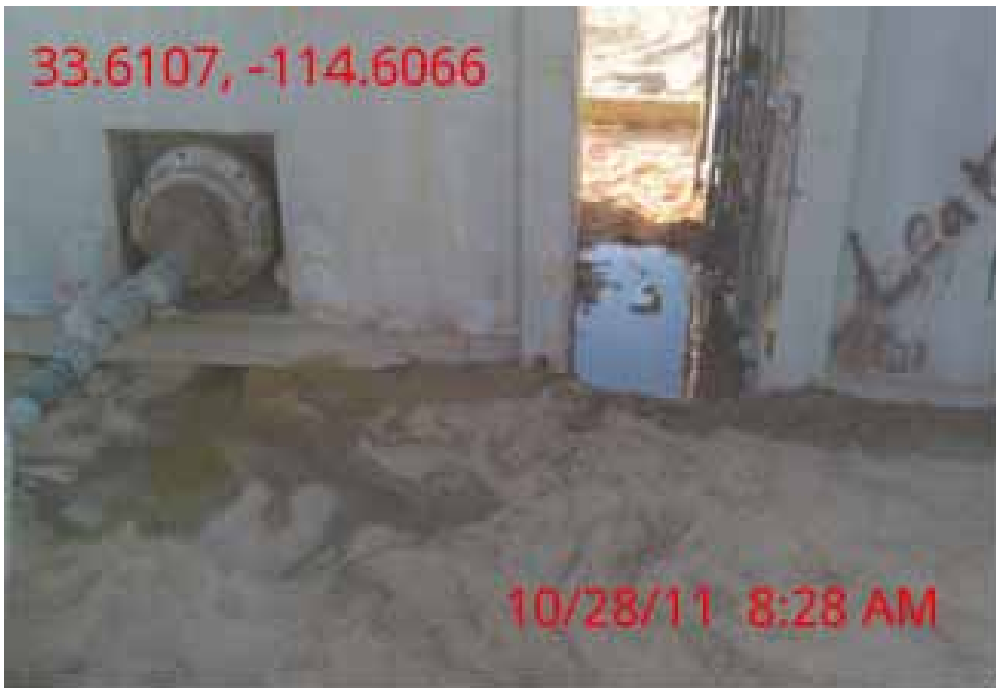
Figure 9: Water leaking from Baker tank at CRS site. A hose was attached to tank to resolve any erosion issues.
