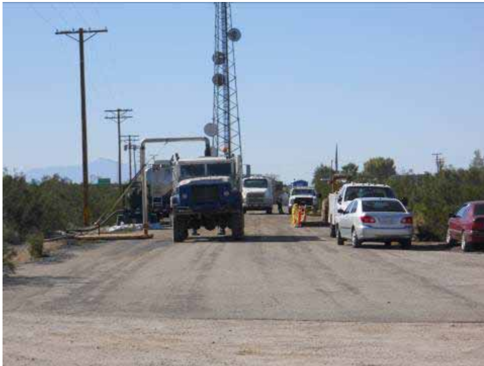
Figure 3: J-stand water tower installed along access road south of Summit Construction Yard. A verbal warning was issued by the CPUC EM because this was not an approved water source location.
