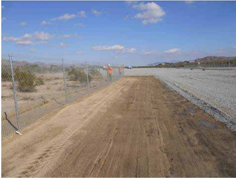
Figure 1: Fence installation, grading, and gravel placement activities occurring at the Summit Construction Yard.
