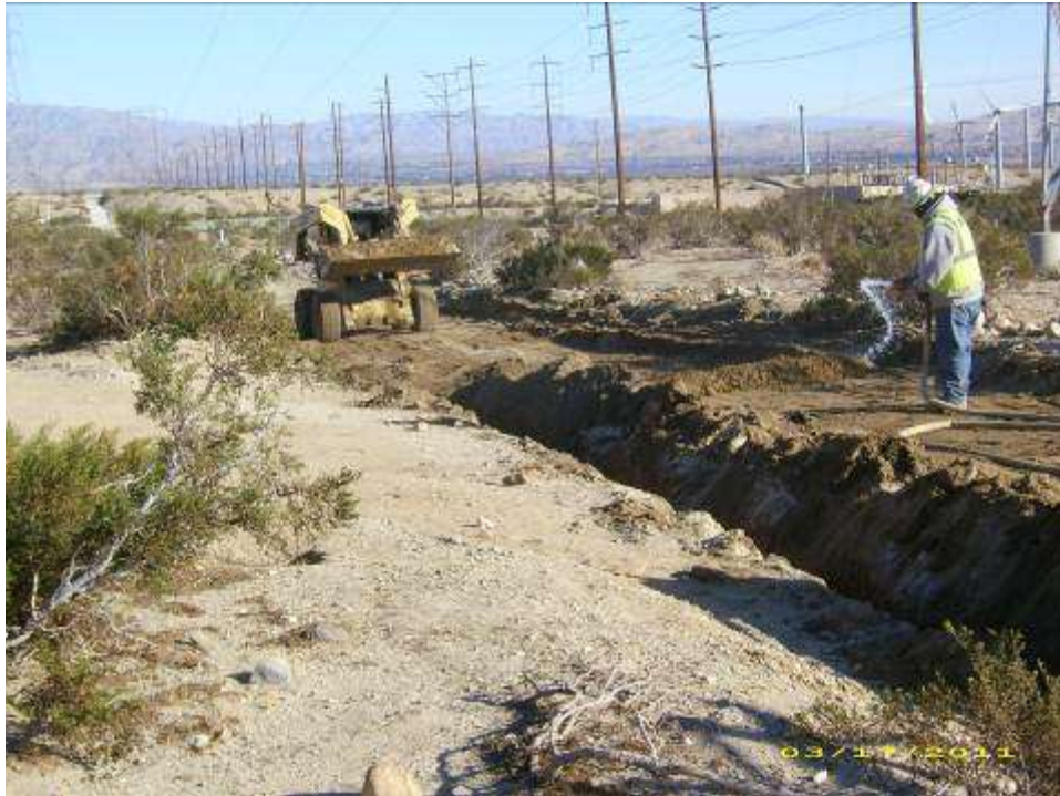
Figure 1: Major construction activities associated with the underground temporary power at the Devers #1 Construction Yard.
