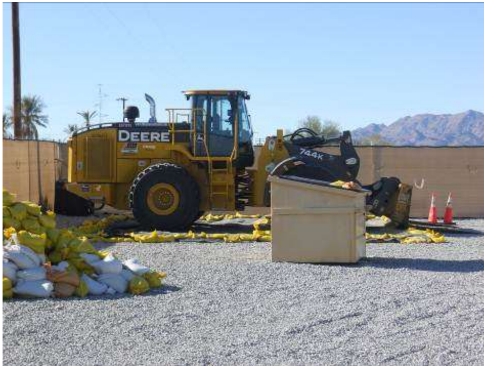
Figure 2: Heavy equipment parked on plastic sheeting and secured trash containers at the Desert Center #1 Construction Yard.
