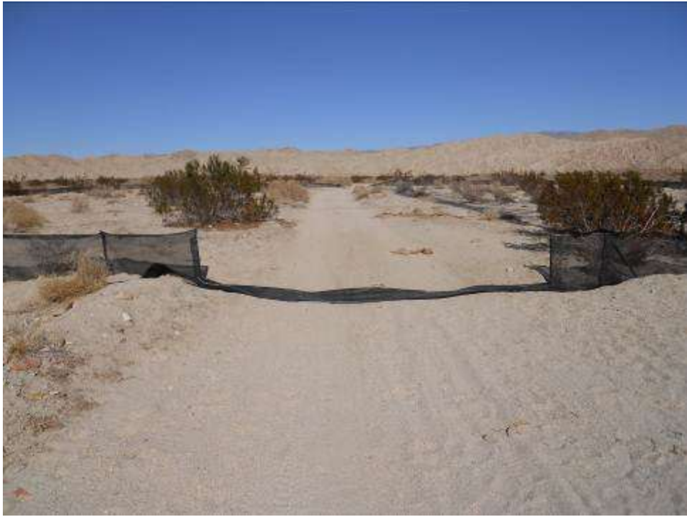
Figure 5: Damaged exclusionary fencing at entrance gate and along back northern boundary at Tower #2133.
