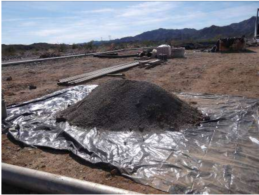
Figure 7. Contaminated gravel placed on plastic sheeting at Red Bluff Substation.
