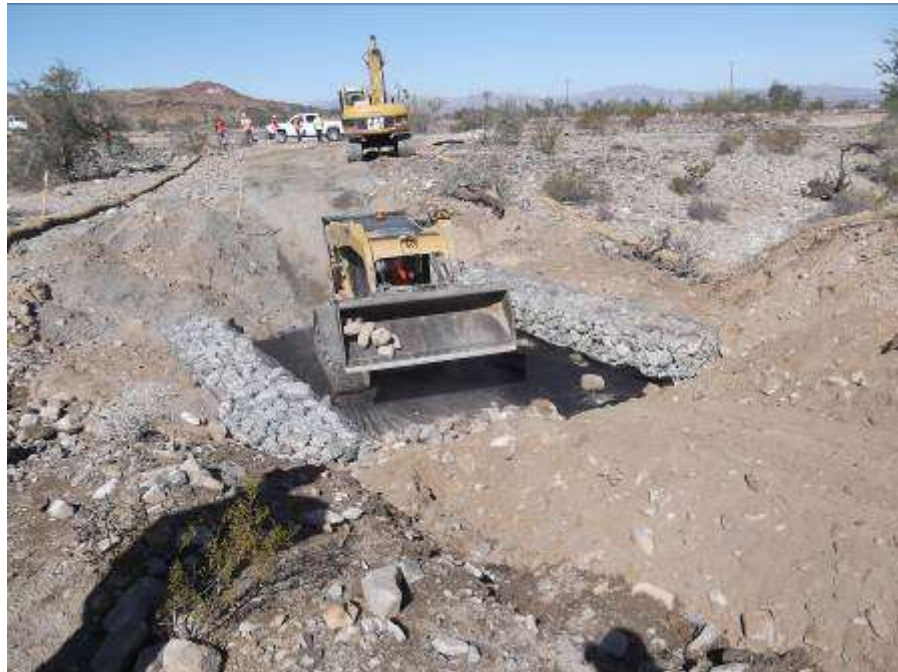
Figure 2. Construction of a wet crossing along the spur road to Tower RB1-4E.
