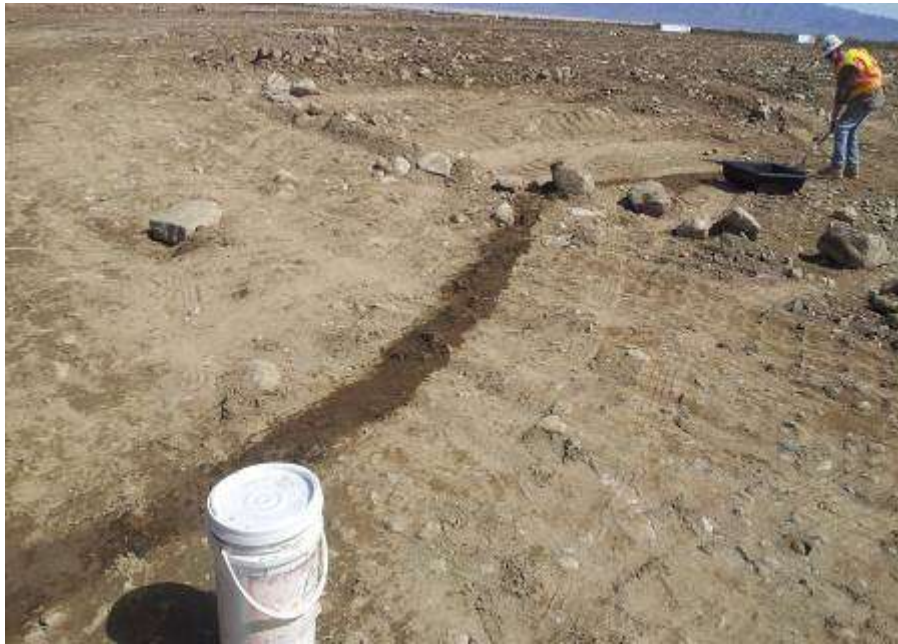
Figure 7. Fuel leak and containment efforts at Red Bluff Substation site.
