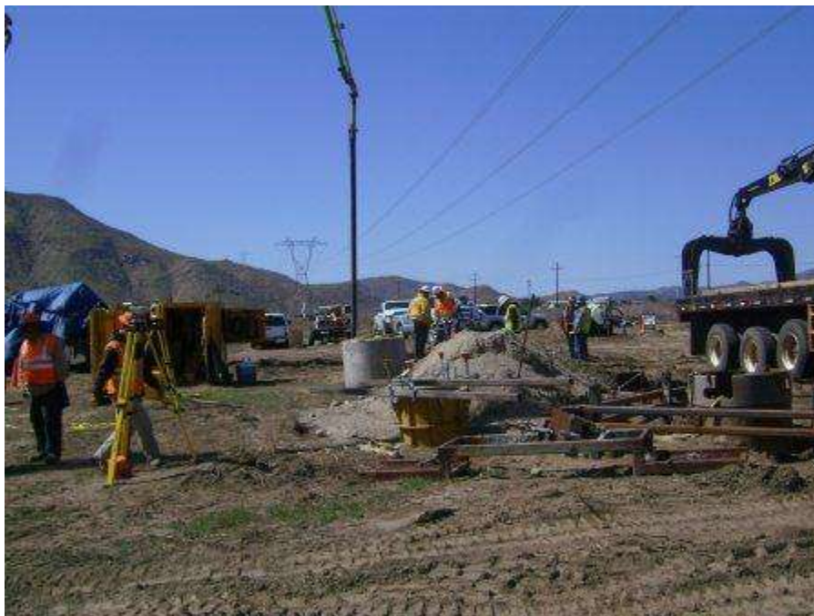
Figure 6. Foundation concrete pouring occurring at Tower 1060 within the 300ft ESA buffer for an active common raven nest.
