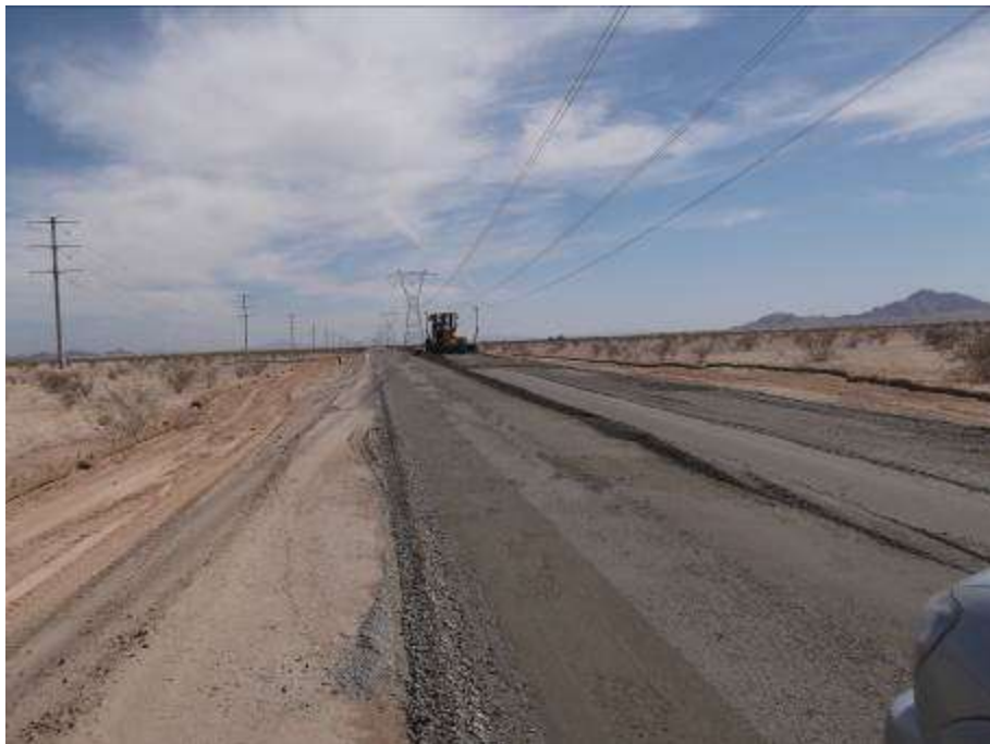
Figure 8. Installation and grading of road base material along CRS primary access road.
