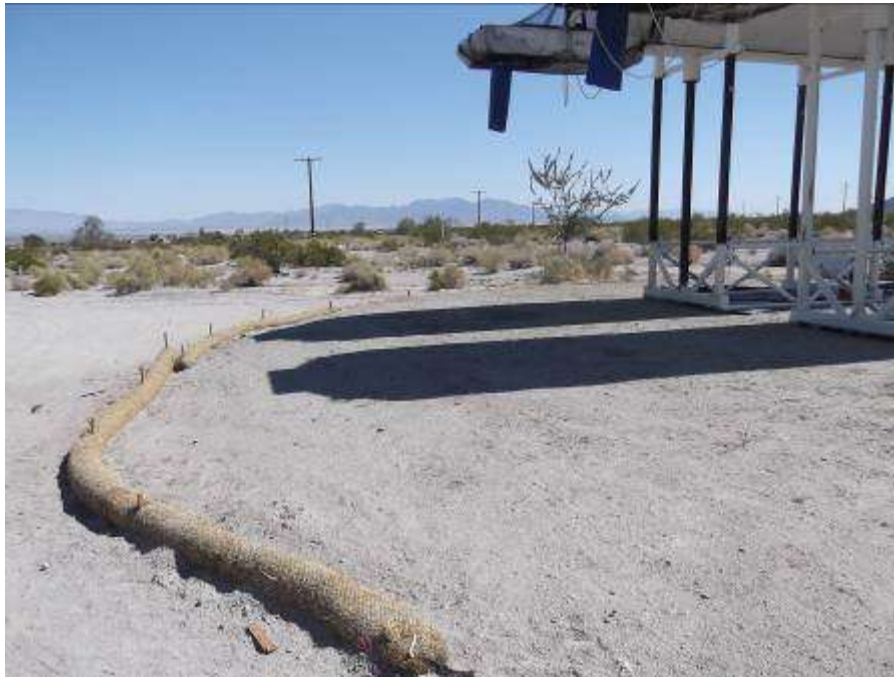
Figure 5. BMPs and bird netting installed at water stand tank at Rice Road location.
