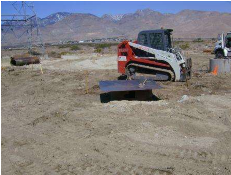
Figure 7. Covered foundation hole with a gap where animals could potentially fall into.
