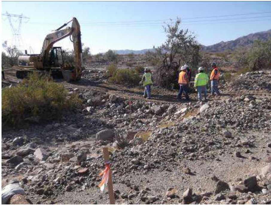
Figure 3. Construction of wet crossing along spur road to Towers RB1-5E and RB2-5E.
