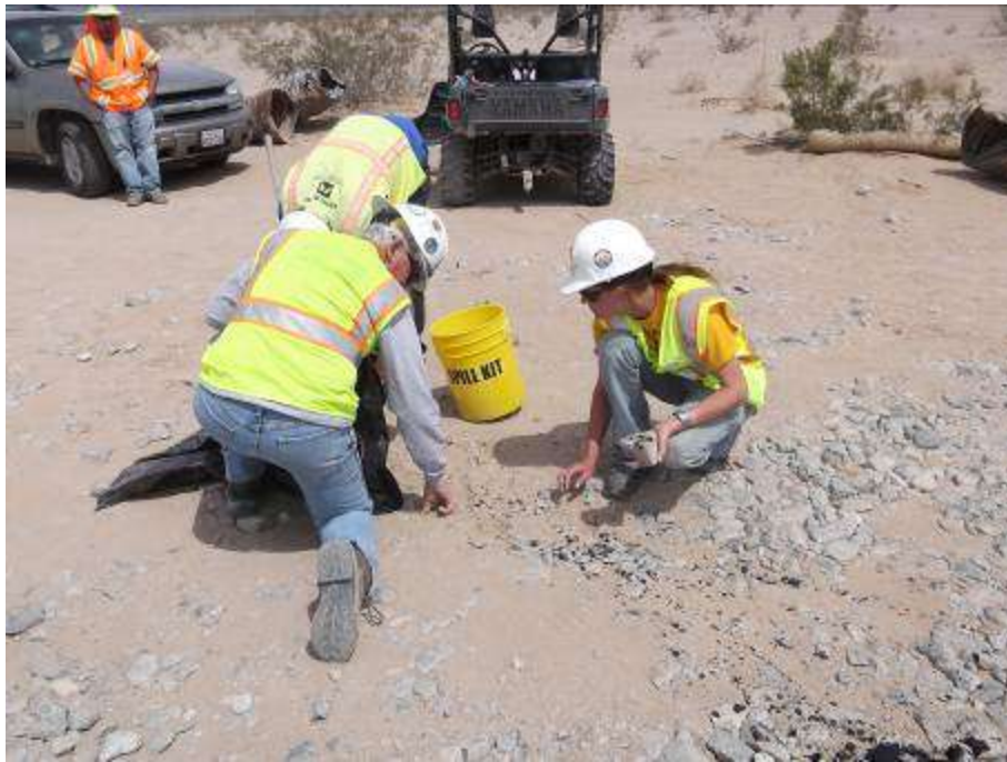
Figure 9. Construction and monitoring personnel removing contaminated soil and rocks from asphalt emulsion spill site along CRS access road.
