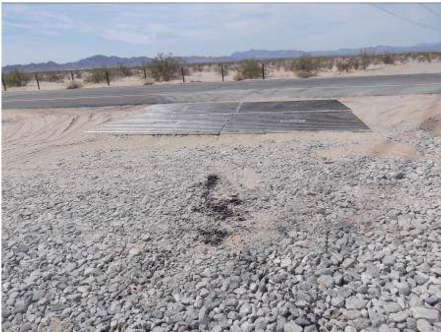
Figure 8. Asphalt emulsion spill scattered along CRS access road near ingress/egress.
