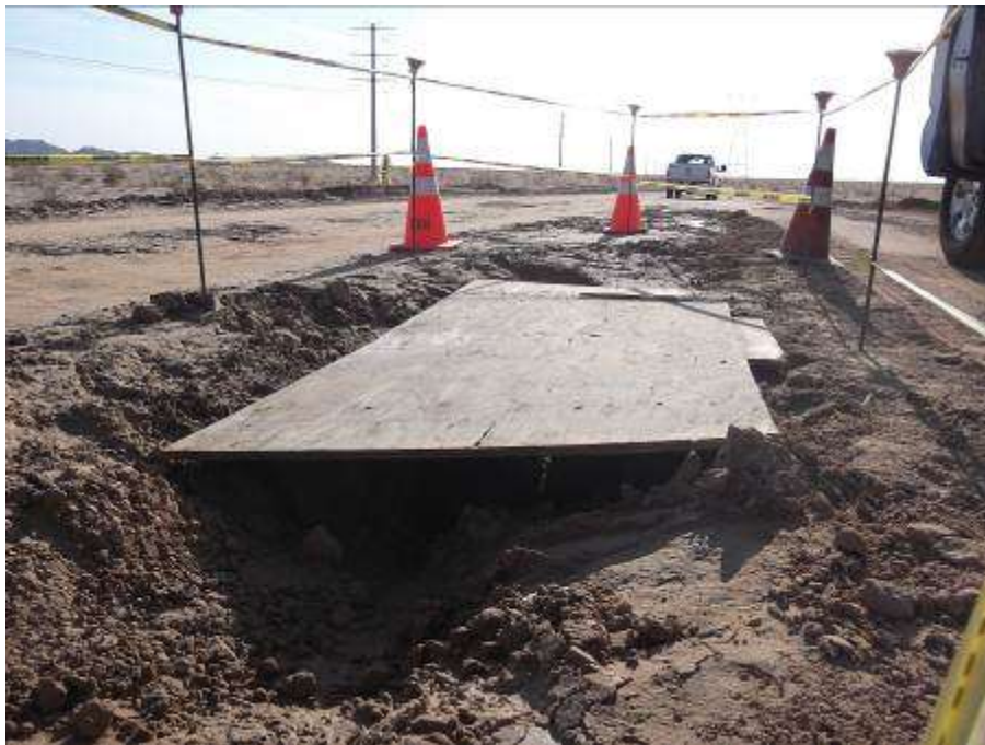
Figure 8. Inadequate trench covering observed by CPUC EM along CRS primary access road.
