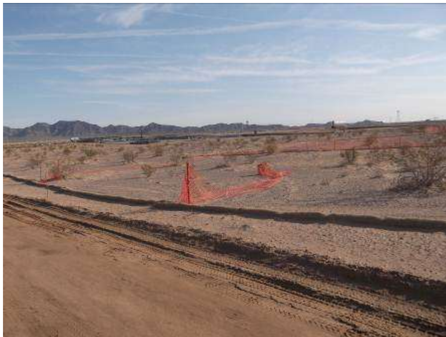
Figure 4. Damaged ESA fencing along CRS Loop-In access road.
